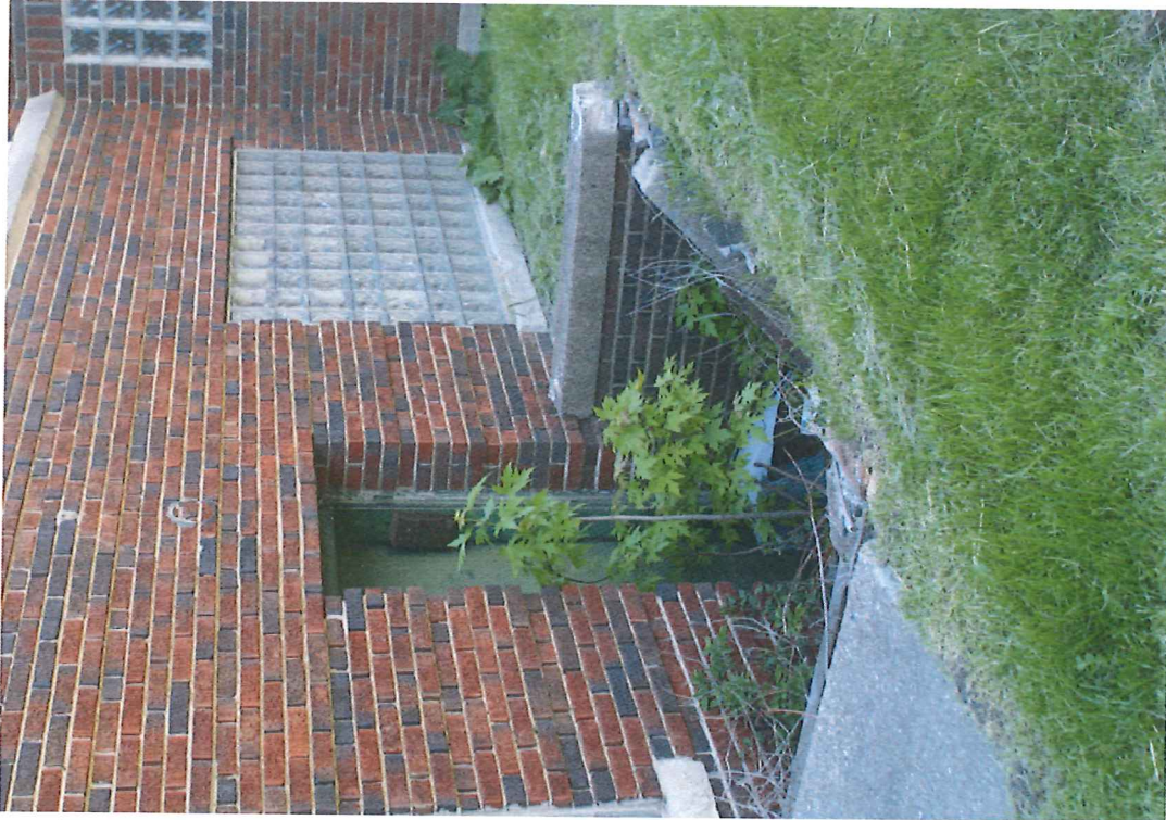
Supplemental Photo A: Exterior View, West Elevation, Retaining Wall to Basement Door
