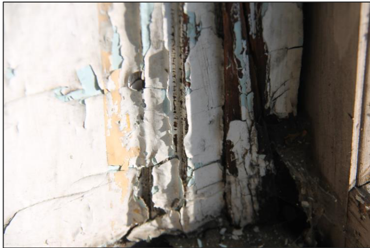
Rotted jamb behind board-up that was removed
