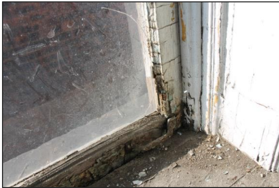
Failed Corner Joinery, Bottom Rail
