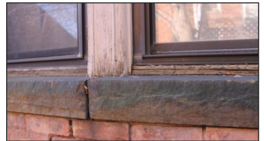
1 st floor window, viewable sill condition - poor
