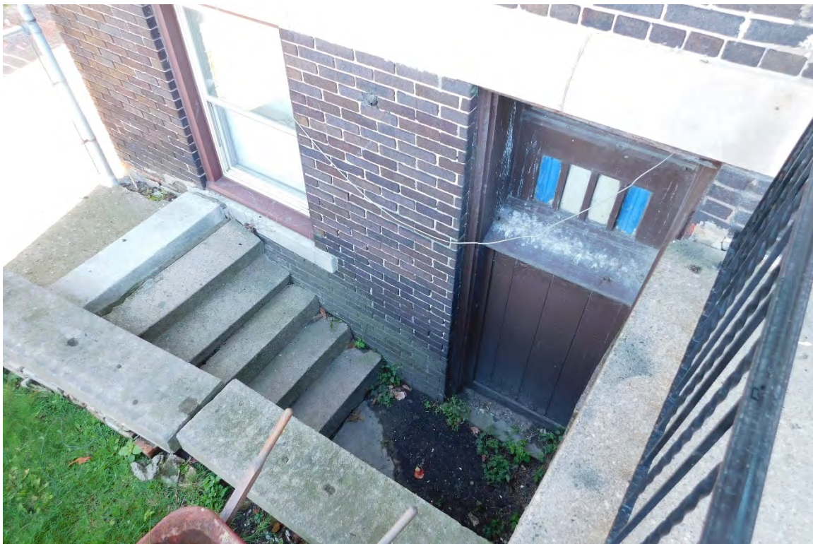
Figure #07: Exterior, Eastern side of North façade, Exterior access to basement, Looking Down. 10/28/20.
