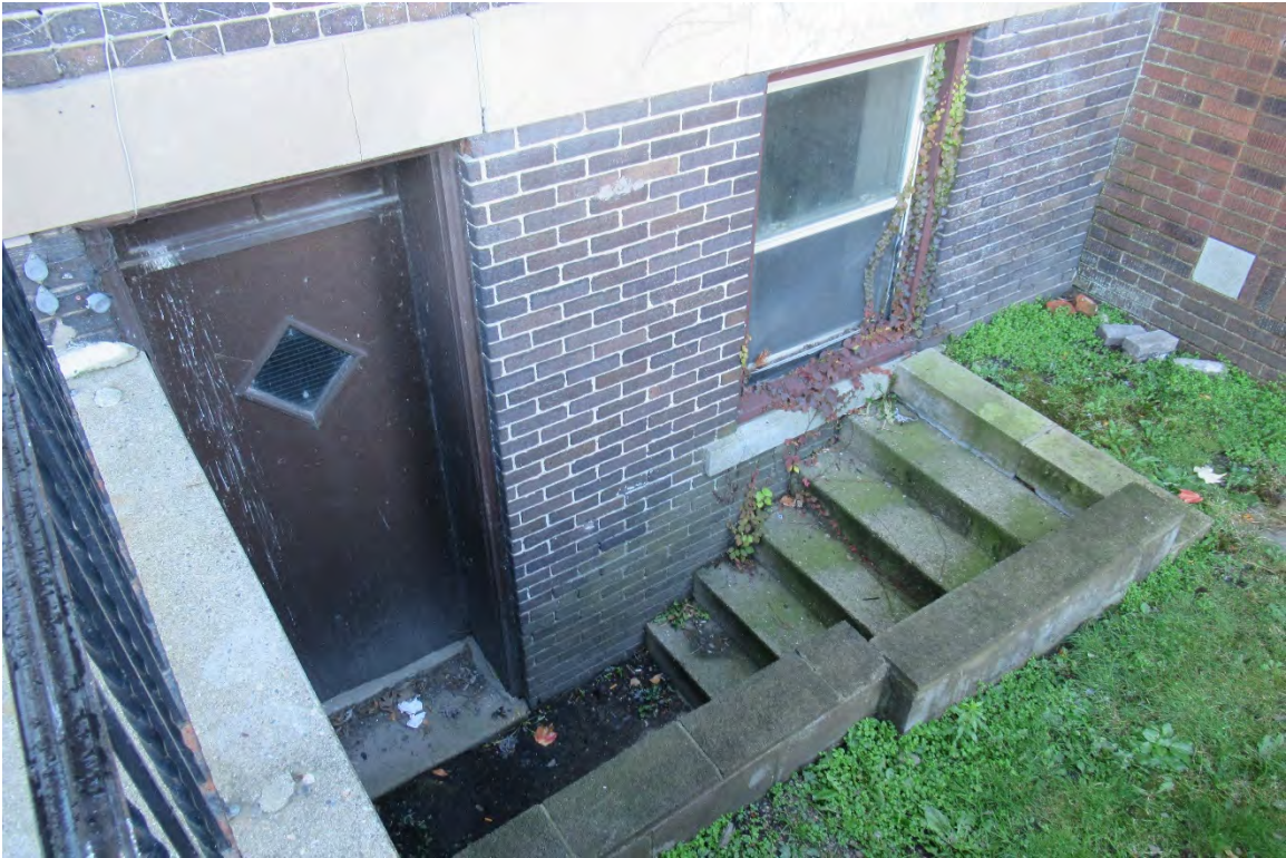
Figure #08: Exterior, Western side of North façade, Exterior access to basement, Looking Down. 10/28/20.
