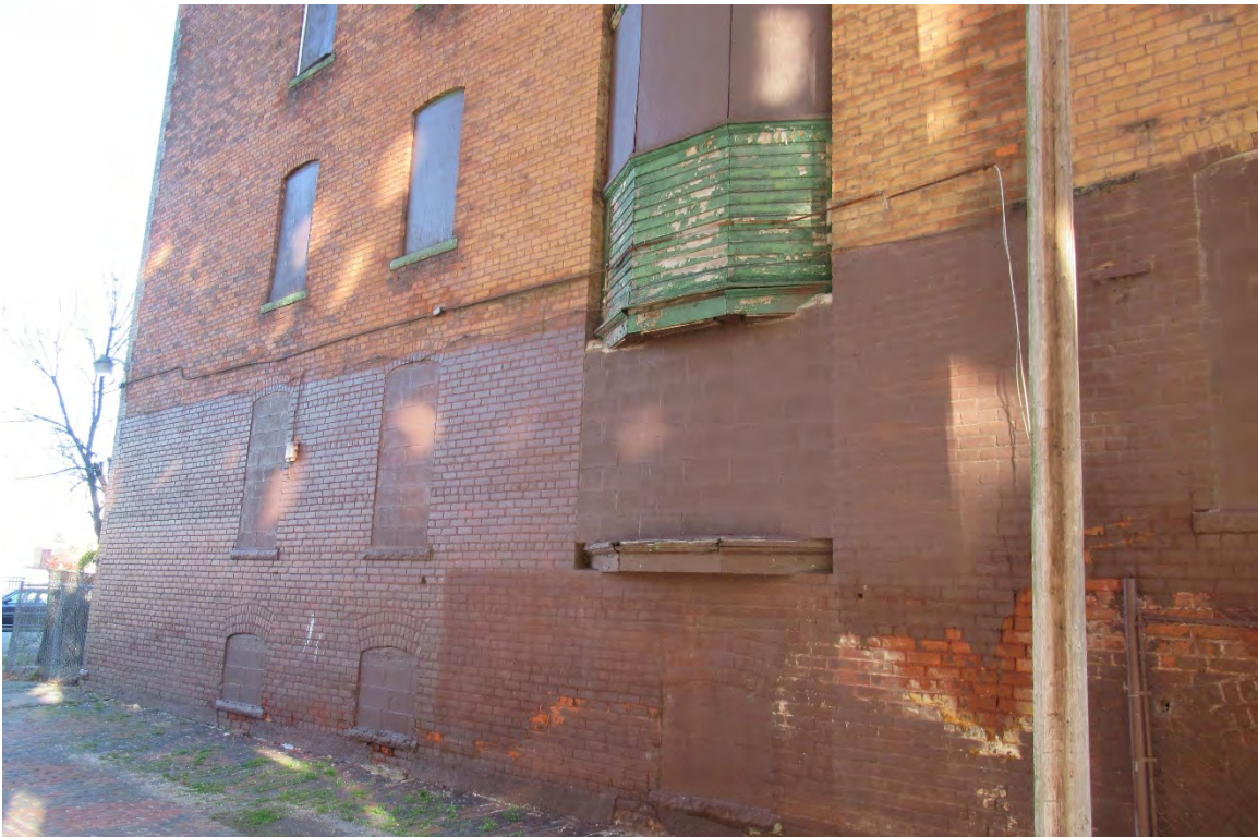
Figure #15: Exterior, West façade masonry infilled first floor bay window detail, Northeast. 10/28/20.
