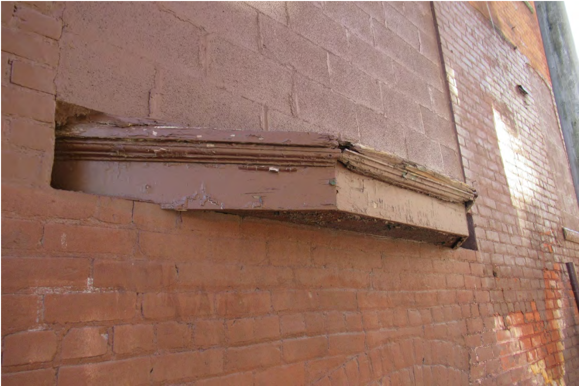
Figure #16: Exterior, West façade masonry infilled first floor bay window detail, Looking Southeast. 10/28/20.
