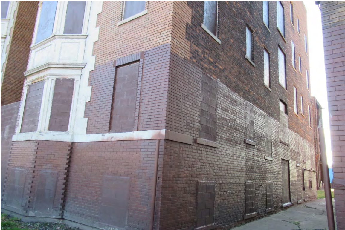
Figure #21: Exterior, Western edge of North façade and West façade, Looking Southeast. 10/28/20.
