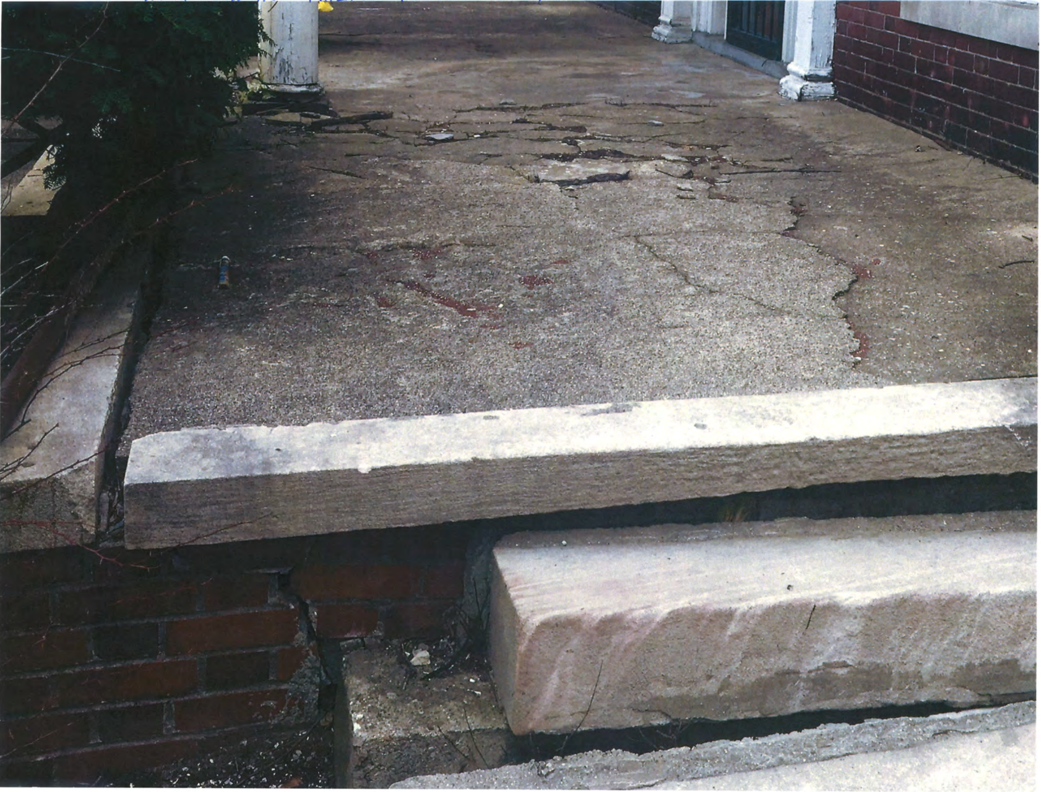
1991 CHICAGO FAILING PORCH 2017
