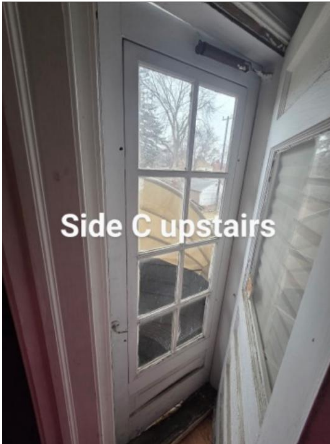
Interior of the rear balcony storm door and the exterior of the rear balcony entry door. Some wood deterioration can be observed below the glass on the storm door. These doors are identified as "11" by staff.
