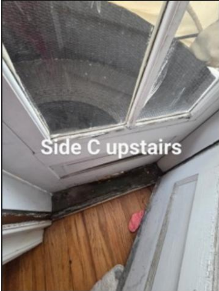
Rear balcony storm door interior and entry door exterior. Some deterioration can be seen in the wood below the glass on the storm door. Staff identified these doors as "11."
