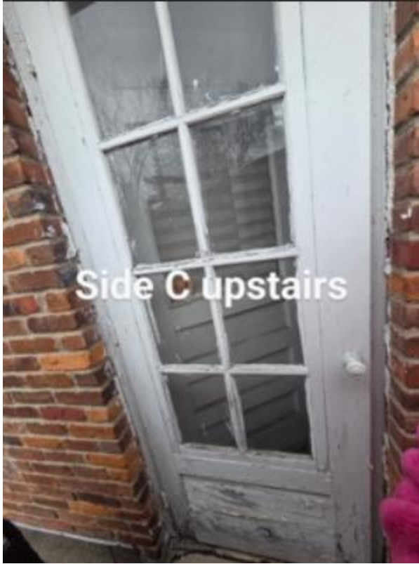
Exterior of the rear balcony's storm door. Some wood deterioration is evident below the glass. Staff identifies this door as "11."
