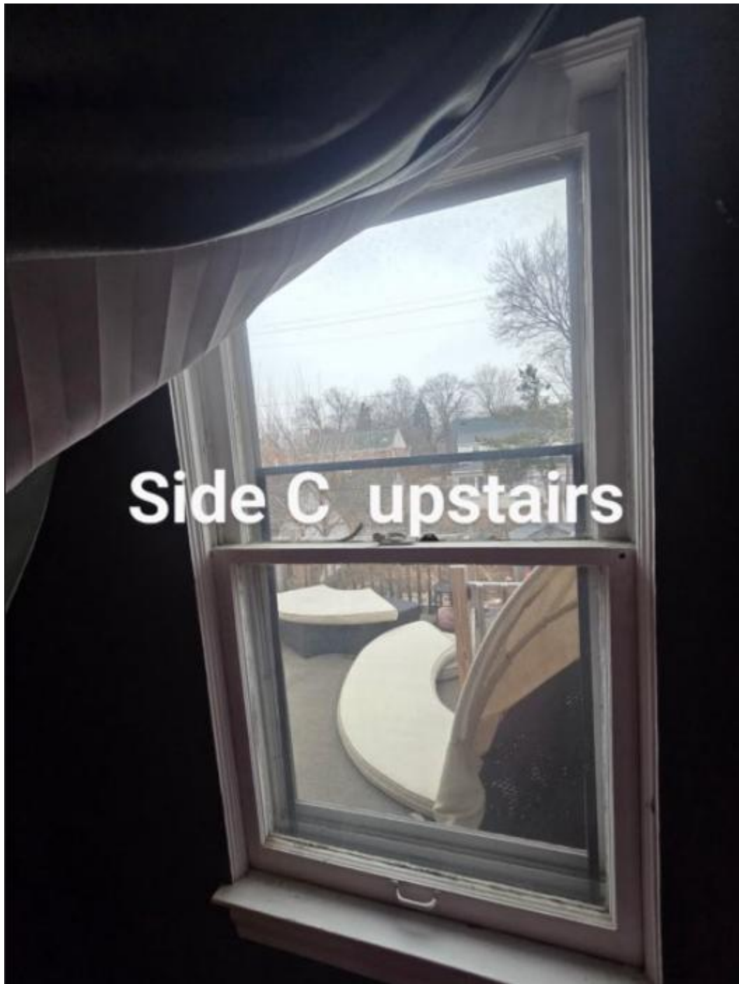
Staff identified this window as Window 12 . It appears to be a wood window without muntins. Staff believes this to be a wood replacement window.
