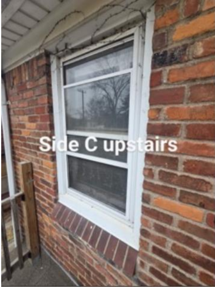
Window 10 by staff's identification. This appears to staff to be a replacement window.
