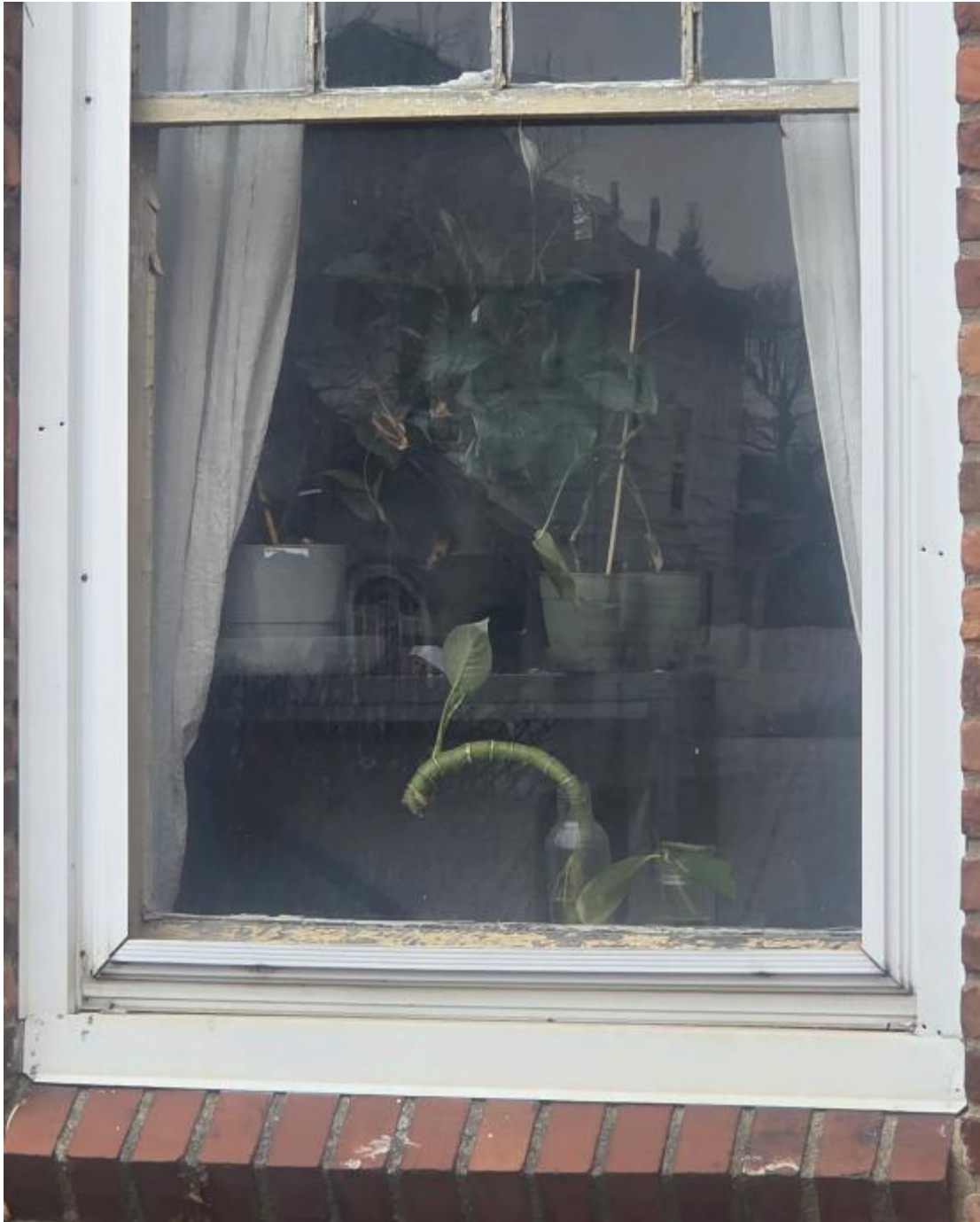
In the Cycle 3 application materials, this window was identified as “Living room 2A,” and the photo was high resolution, so staff included this image of the lower sash. Staff identifies this window as Window 5 .
