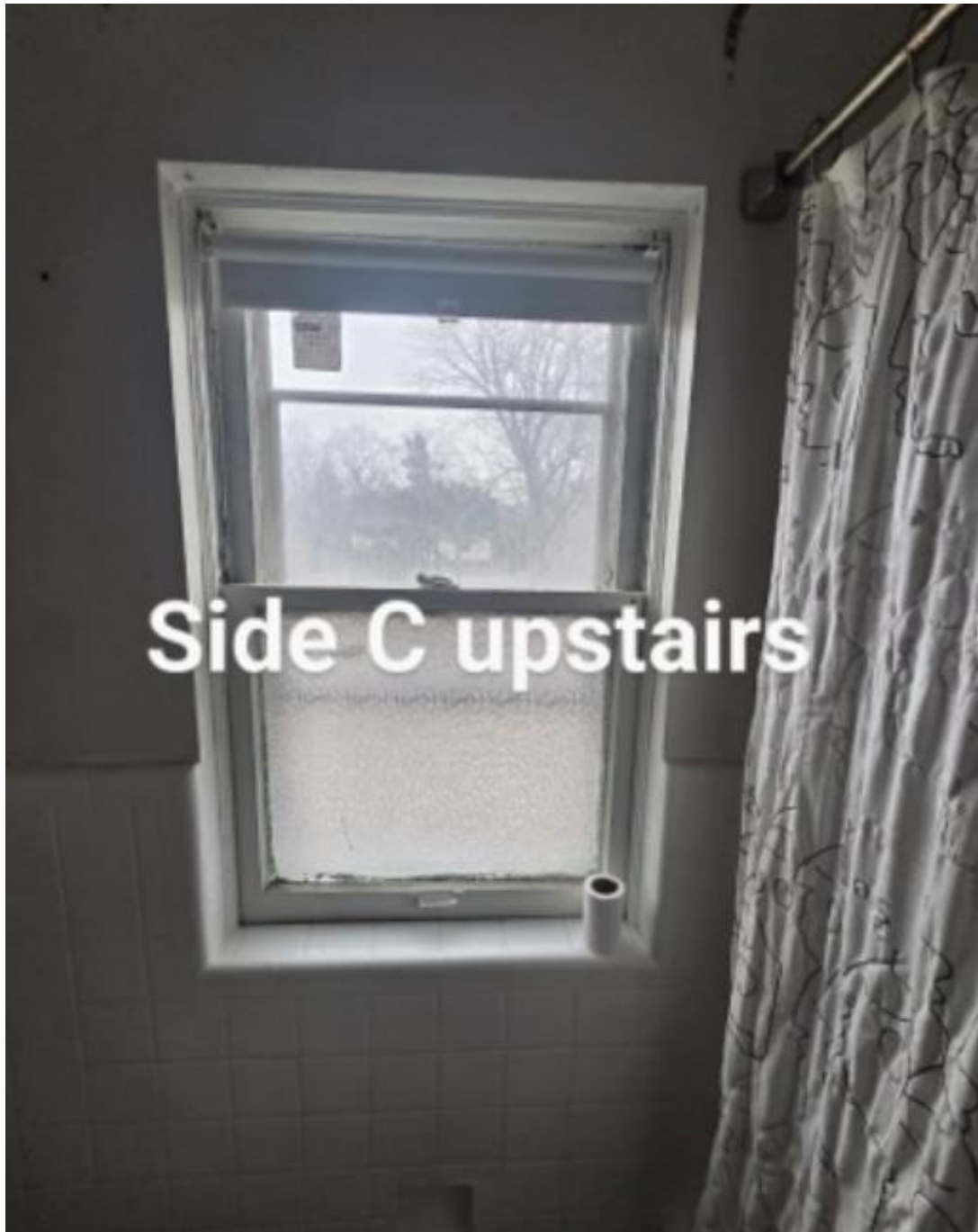
Window 10 by staff's identification. This window appears to staff to be a wood replacement window.
