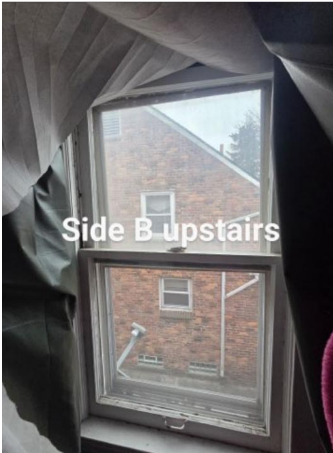
Side B upstairs windows correspond to staff's Windows 6 or 7. Based on the arm of the satellite dish being visible here, staff believes this to be Window 6 . It appears to be a wood replacement window.
