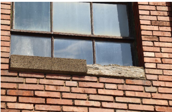
Staff photo, Existing Cast Stone, 04/22/26
