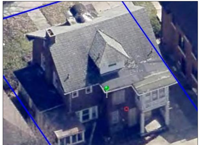
This aerial view confirms the porches and windows at the enclosed second floor rear porch remained intact. ConnectExplorer, April 2024
