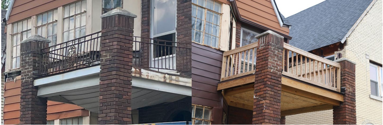
Photo taken by staff on 06/24/24, for a violation for roof rehabilitation.
