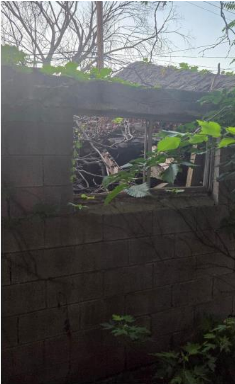
3768 Tyler, garage, south wall, applicant-provided photo from materials. Currently, there is no roof on this portion of the structure. The applicant's drawing shows this south wall with a gable roof, but if the garage is to be rebuilt as it was, the peak of the gable roof would be centered over the east and west sides instead.
