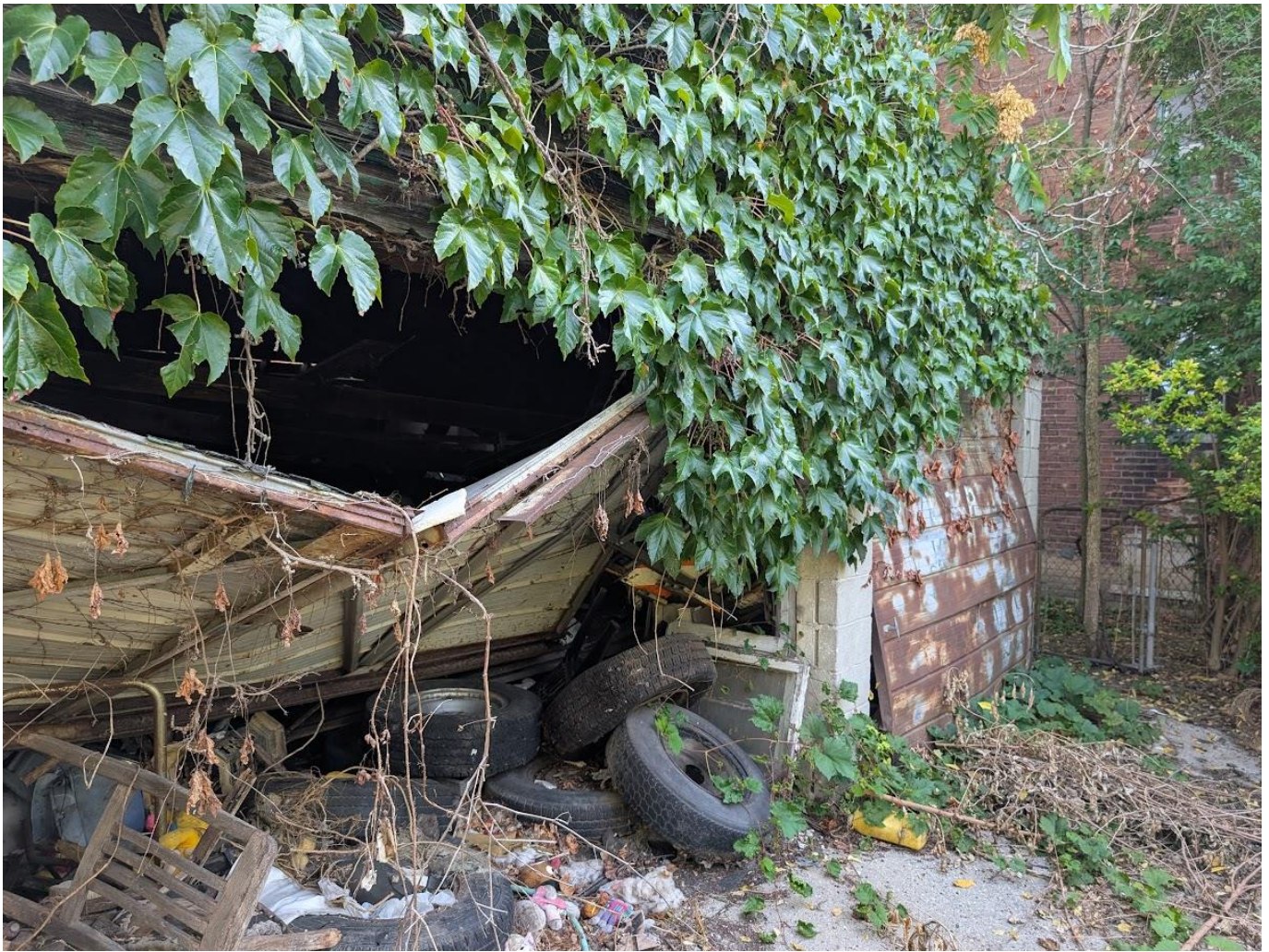
3768 Tyler, garage, west side from near the northwest corner looking toward the southwest corner. The non-collapsed garage door is at the southwest corner. These overhead doors were shown in the 2006 aerial photo, before the roof collapse. Applicant has labeled the long sides of the garage on their drawing as "NORTH" and "SOUTH." The applicant's drawing labeled "WEST" has a peak and a garage door, but is clearly a short end of the structure (either the north or south). (Staff site visit, September 2025)
