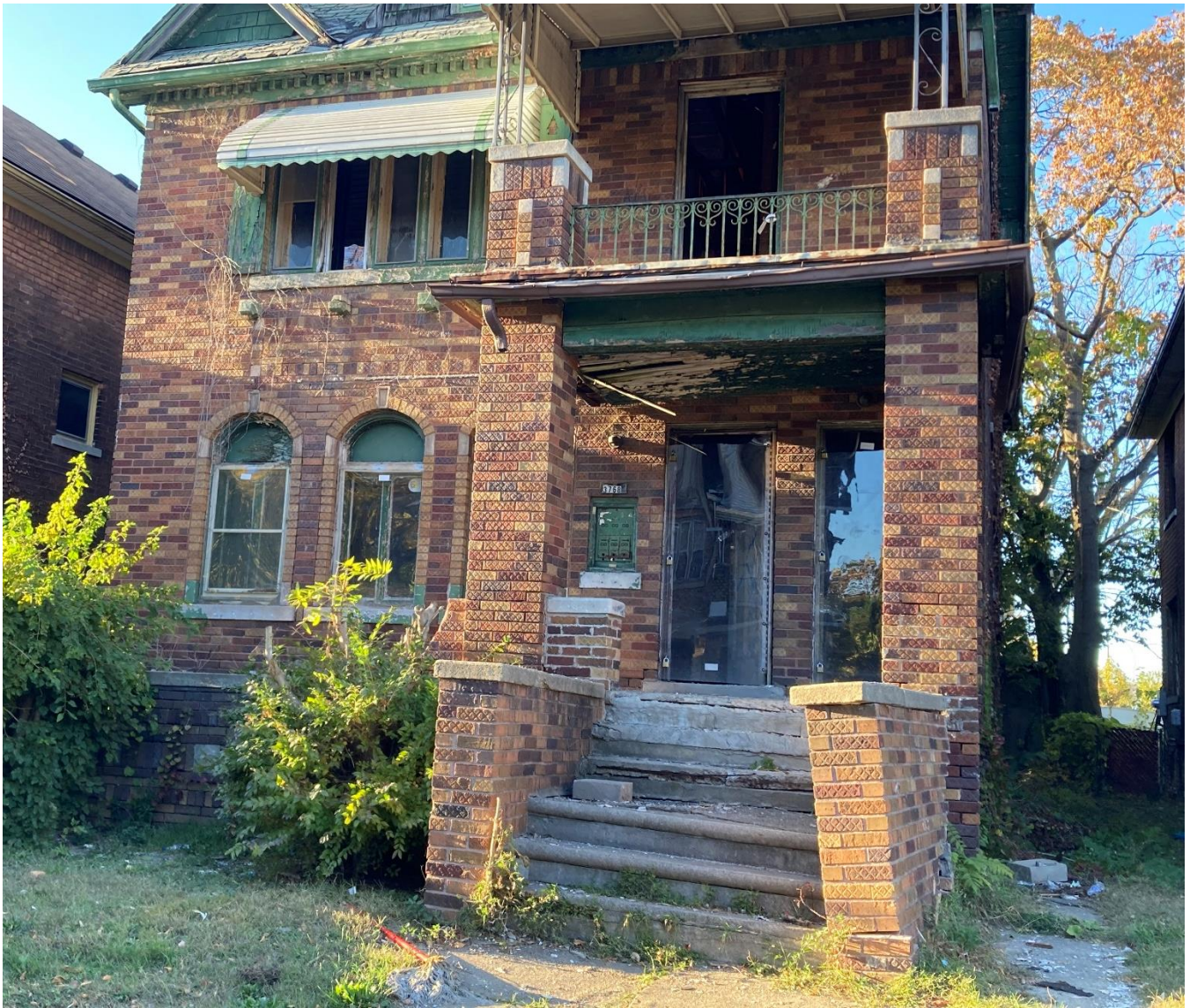
3768 Tyler, south end, staff photo, October 2025. The eastern wing wall next to the front step is leaning and the front steps and porch cap are deteriorated. These conditions will be addressed as part of the approved front porch rebuild, and the porch ceiling will be repaired in kind. New gutters and downspouts, painted to match the wood trim, were also approved. The aluminum awning over the front porch has been removed. The diamond-patterned brick can be seen in the sunlight.
