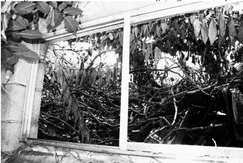
3768 Tyler, garage, south end sliding window, but lacks glass. Applicant plans to repair it and insert new glass, but may ultimately remove the window frame and block in the opening. Because the garage dates from 1966, it is outside the period of significance.
