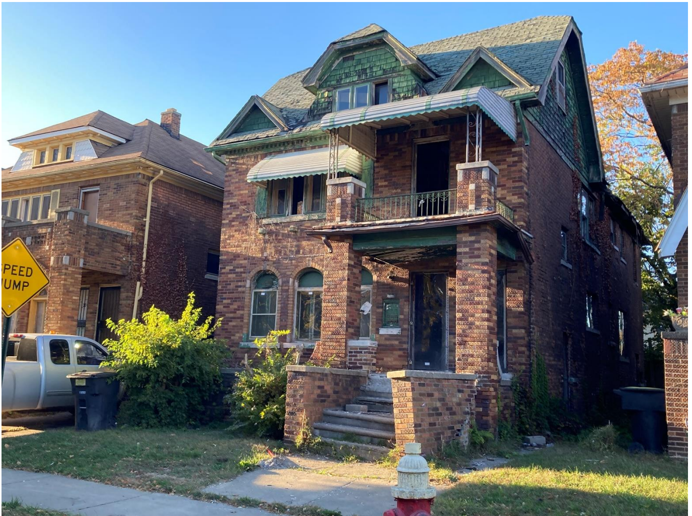
3768 Tyler, south end and east side, staff photo, October 2025. The eastern wing wall next to the front steps is leaning and the front steps and porch cap are deteriorated. These conditions will be addressed as part of the approved front porch rebuild.
