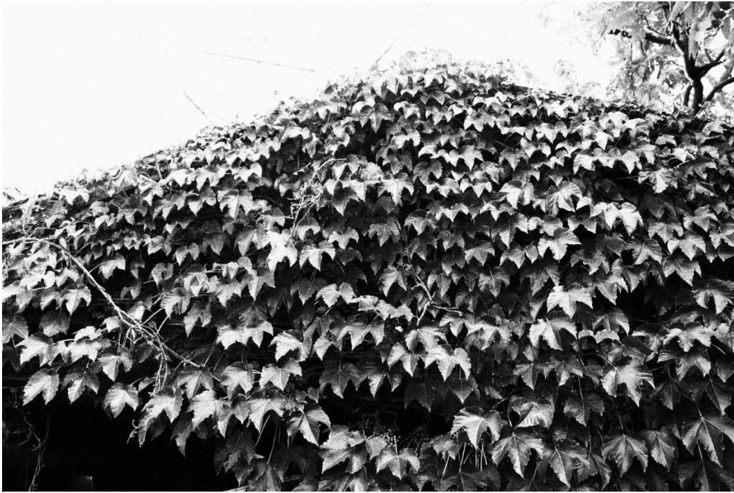
3768 Tyler, garage, extreme overgrowth visible at the peak of the gable on the west side. (Staff site visit, October 2025)
