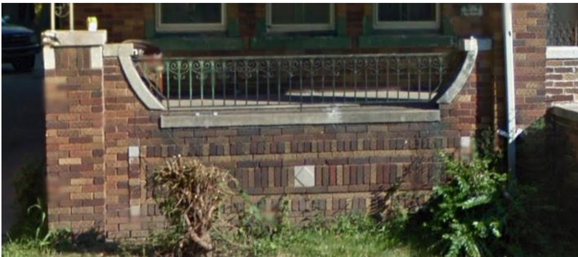
Front porch detail from August 2011, courtesy of Google Street View. Railing is now missing.
