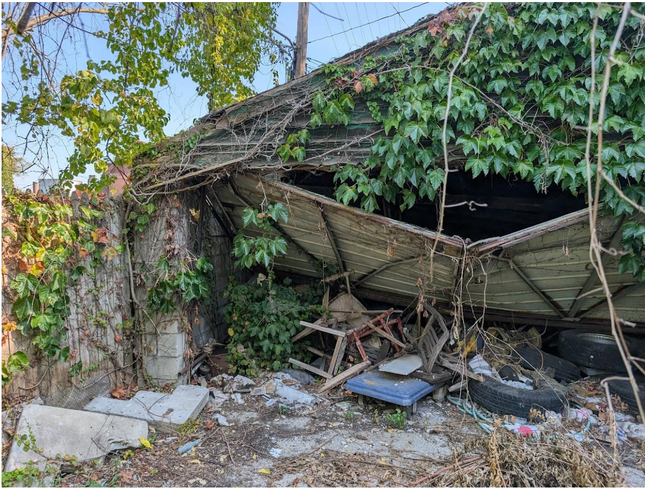
3768 Tyler, garage, west side near the northwest corner. This overhead door was shown in the 2006 aerial photo, before the roof collapse. Applicant has labeled the long sides of the garage on their drawing as "NORTH" and "SOUTH." The applicant's drawing labeled "WEST" has a peak and a garage door, but is clearly a short end of the structure (either the north or south). (Staff site visit, September 2025)
