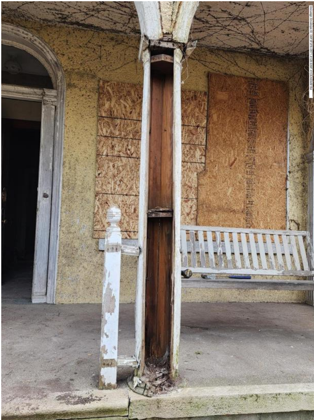
Applicant's photo, April 2025. Porch column half removed, base is in poor condition. Newel post visible to support the handrail for the steps.
