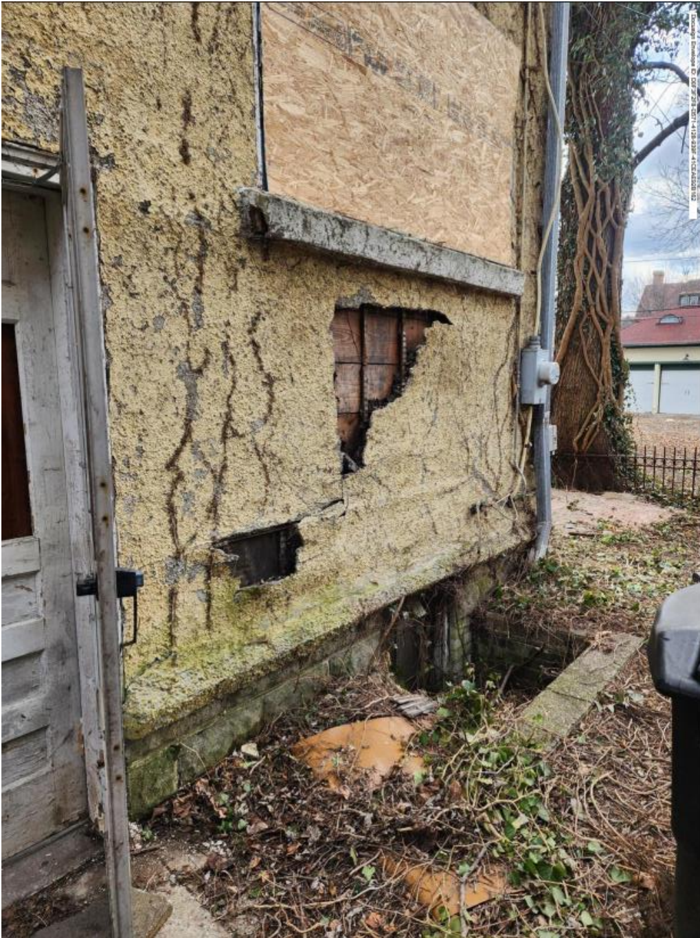
Sample stucco repair needed, applicant photo, April 2025.
