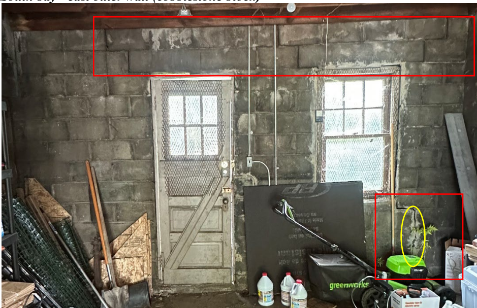
Step cracks above the window and door. Cracked tile below window.
