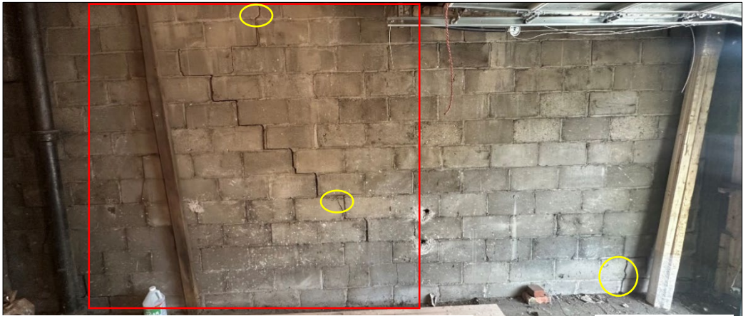
Large step crack, broken blocks at top and near middle of wall
