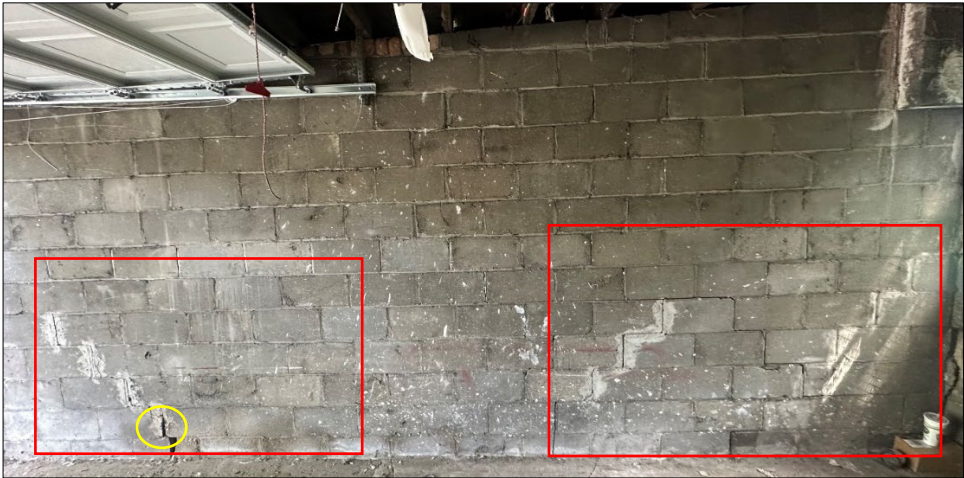
Step crack and cracked block
