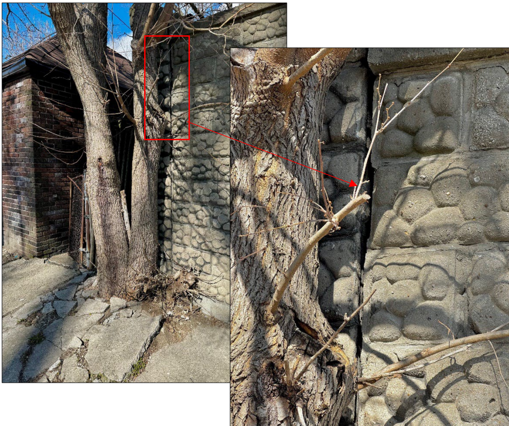
This alternative view of the northwest corner shows how the growth of this tree and its root system caused the pavement to buckle, as well as undermine the stability of the north wall, as it has begun to lean away from the west wall.
