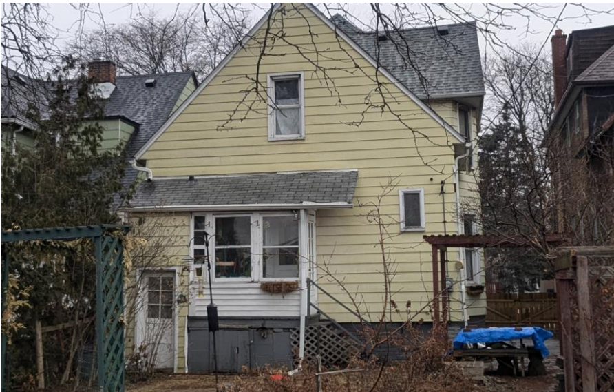
Rear of house viewed from the alley, showing the porch proposed for demolition. February 2025 photo by staff.
