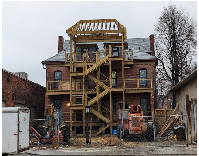
Rear view of 701 West Canfield showing unapproved stair structure and roof form paused during construction, and subject of this application. Staff photo, January 31, 2025.
