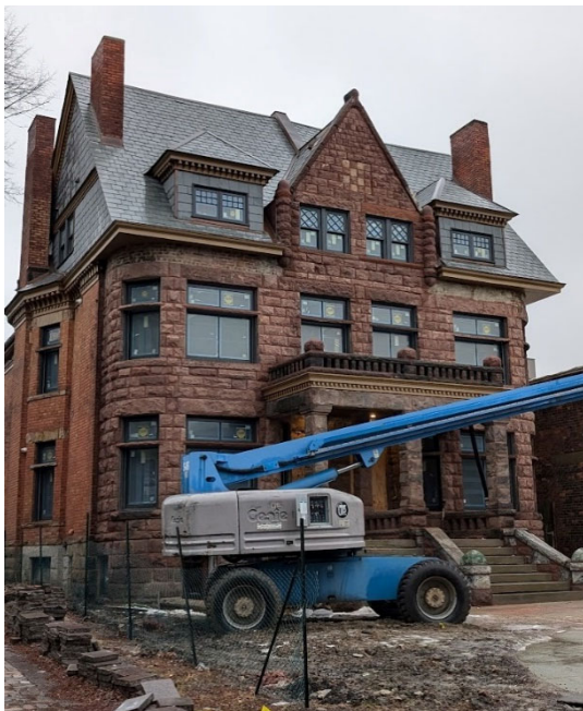
View of 701 West Canfield with approved replacement windows installed. Staff photo, January 31, 2025.
