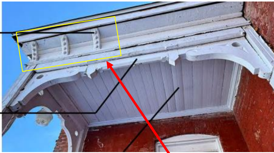
East side porch, current appearance. Note that the east side porch's decorative details match those at the front façade's bay window. Specifically, the brackets at the porch soffit/eave area match those at the front facade bay (outlined in yellow). Provided by applicant as new evidence
