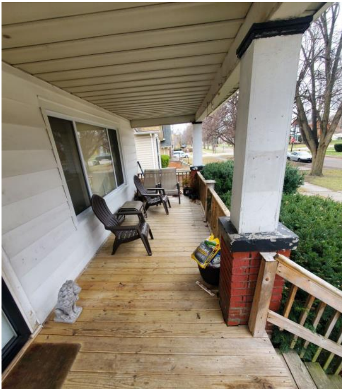
14528 Ashton, facing south. Photo by applicant showing current conditions. Note the wood railing, steps, skirting, and decking which were added without HDC approval in 2016. Also, note the non-historic masonry paver edging at foundation planting
