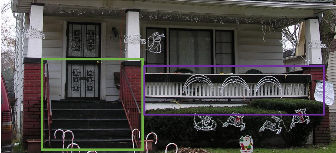
14528 Ashton porch, 2008 designation slide. Source, HDAB. Note the wood guardrails, steps, and flooring. The handrails (outlined in green) are metal while the guardrails (outlined in purple) are wood.
