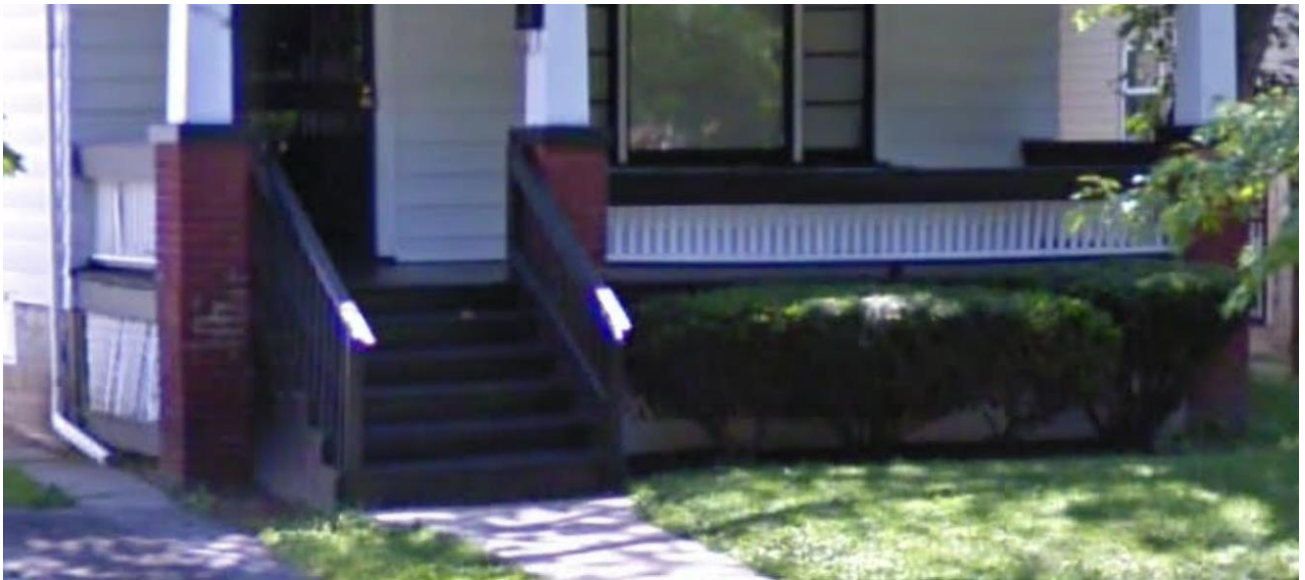
14528 Ashton porch, 2009 appearance. Source, Google Streetview. Note the wood guardrails, steps, and flooring. Also, wood lattice skirting is also visible. However, the metal handrails have been replaced with wood handrails by this point.
