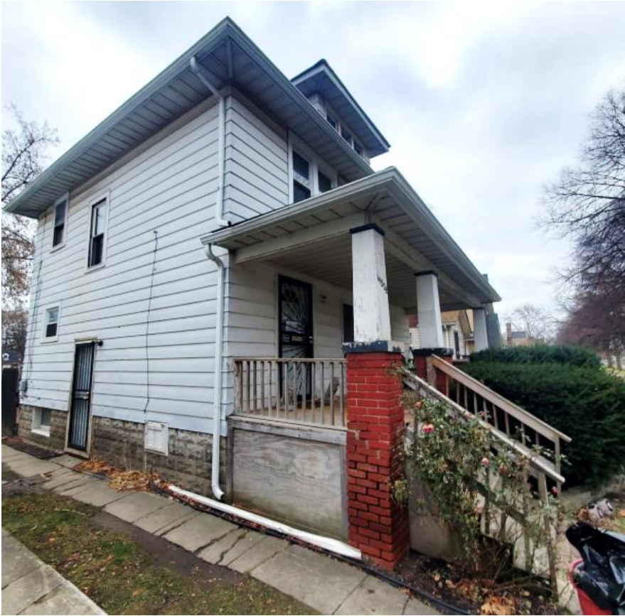
14528 Ashton, facing southeast. Photo by applicant showing current conditions. Note the wood railing, steps, skirting, and decking which were added without HDC approval in 2016.
