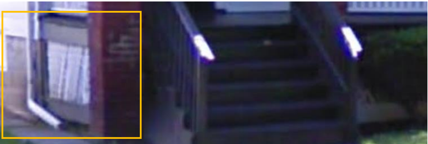
14258 Ashton, Google Streetview image, 2009. This wood lattice skirting (outlined in orange) was replaced without HDC approval in 2016.
