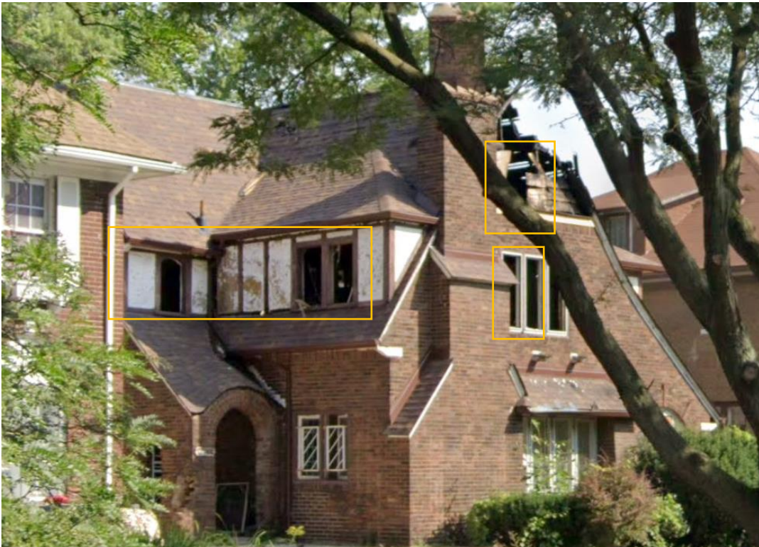
August 2018, after the fire. Window sash outlined in orange appear completely destroyed while their associated trim/casing/ remains. The rest of the windows also remain. Source, Google Streetview
