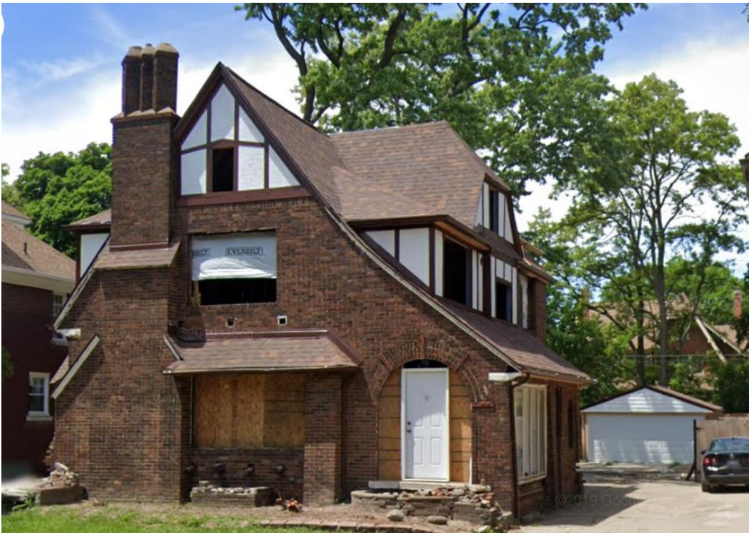
After the fire, 2019. Note that the second and attic story have been rebuilt, most windows and associated casing/brickmould have been removed to the rough opening, and front door sidelites have been removed. Garage siding has also been replaced per the 2018 COA. Source, Google Streetview
