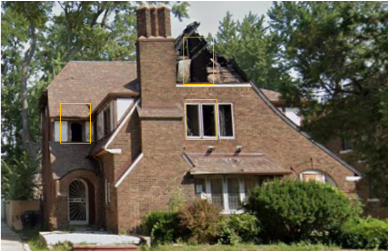
August 2018, after the fire. Window sash outlined in orange appear completely destroyed. The rest appear to remain. Source, Google Streetview
