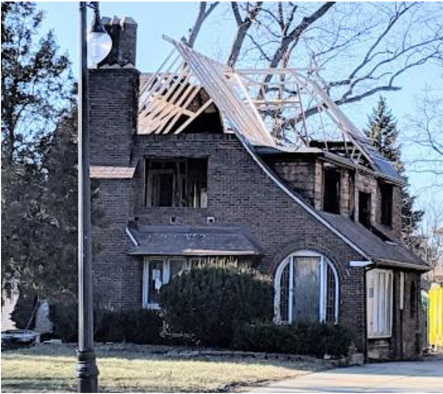
Late 2018, after the fire. Note that the rebuilding of the attic story is underway and all windows and associated casing/trim have been removed at the second story without HDC approval. Source, HDC files
