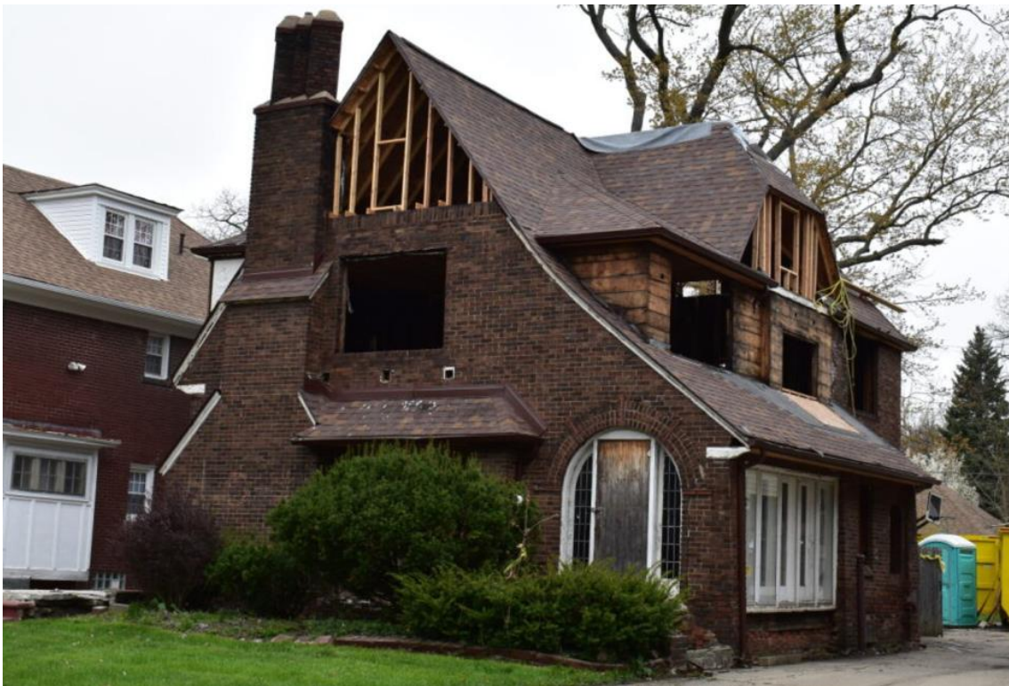
Late 2018, after the fire. Note that the attic story has been rebuilt without HDC approval. Source, HDC files
