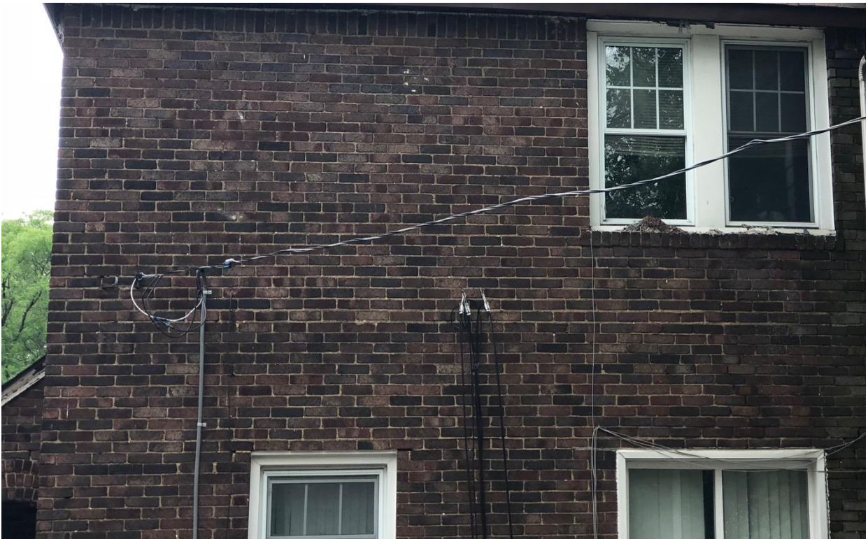
Rear wall, after the 2018 fire. Note that these windows are noncompatible, non-historic vinyl units. Photo from applicant
