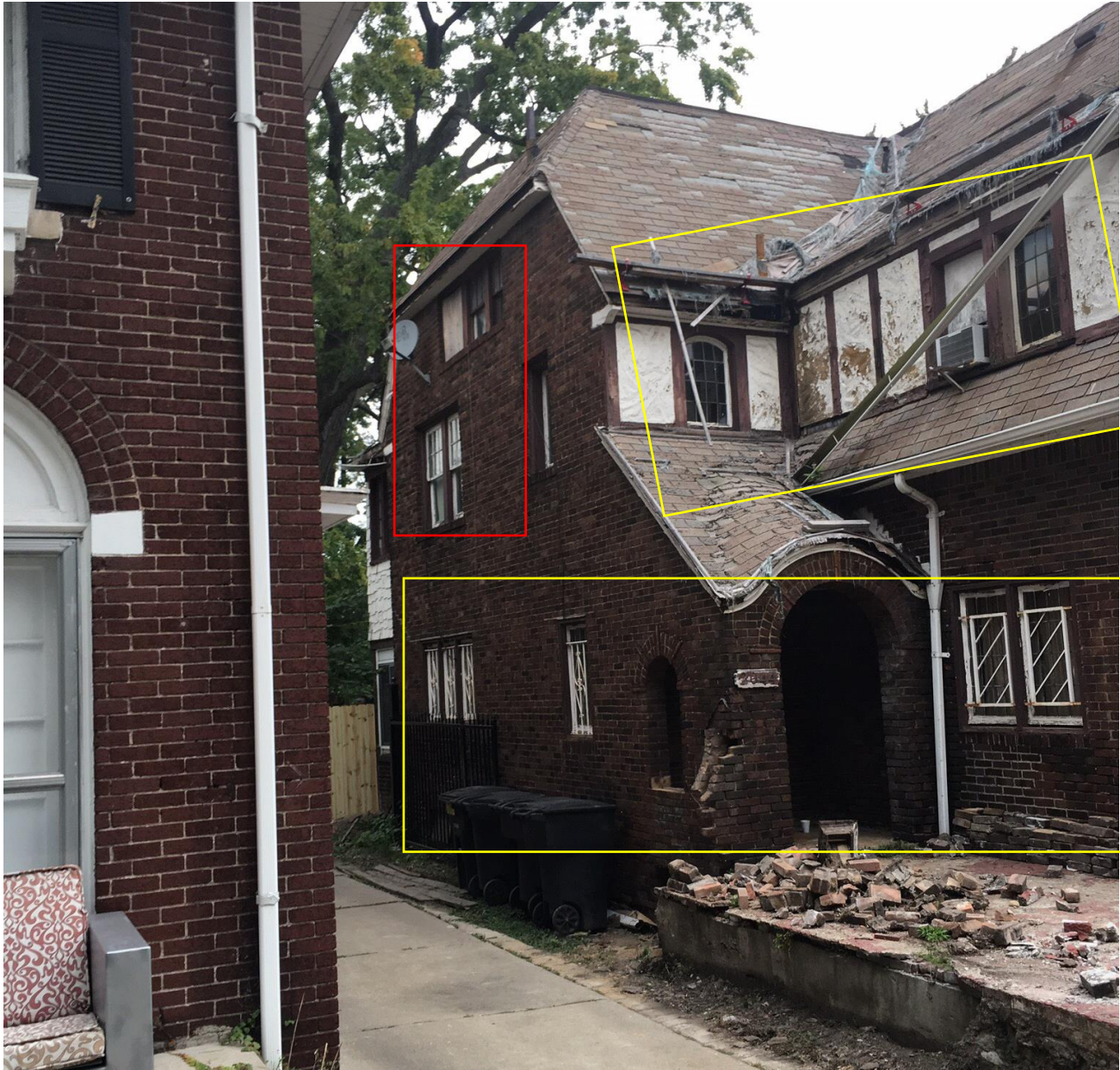
Photo taken in early 2018, prior to the fire. Note that all windows outlined in yellow are wood casement windows with leaded glass and those outlined in red are wood, double hung units. Source, HDC files.
