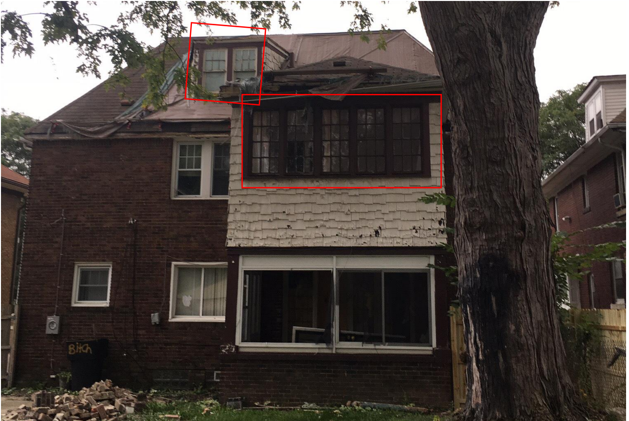
Photo taken in early 2018, prior to the fire. Wood sash casement windows outlined in red. Remaining windows are vinyl. Source, HDC files
