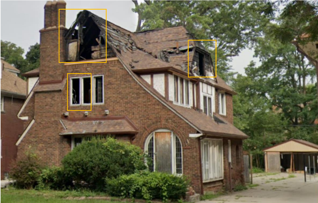
August 2018, after the fire. Note that most of the fire damage appears to be localized at the attic story and second story, west side. Windows sash and trim/casing at attic story outlined in orange appear completely destroyed. Two of the three casement window sash at the front façade, second story (outlined in orange) appear to be completely destroyed although the casing/trim remained. The rest appear to remain. The garage also appears not to have been fire damaged. Source. Google Streetview
