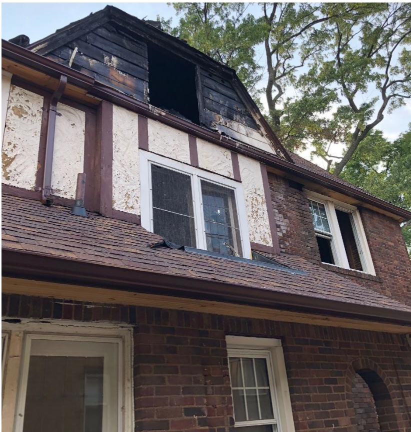
August 2018, after the fire. Detail of fire damage at rooftop dormer, east side. Photo by applicant.
