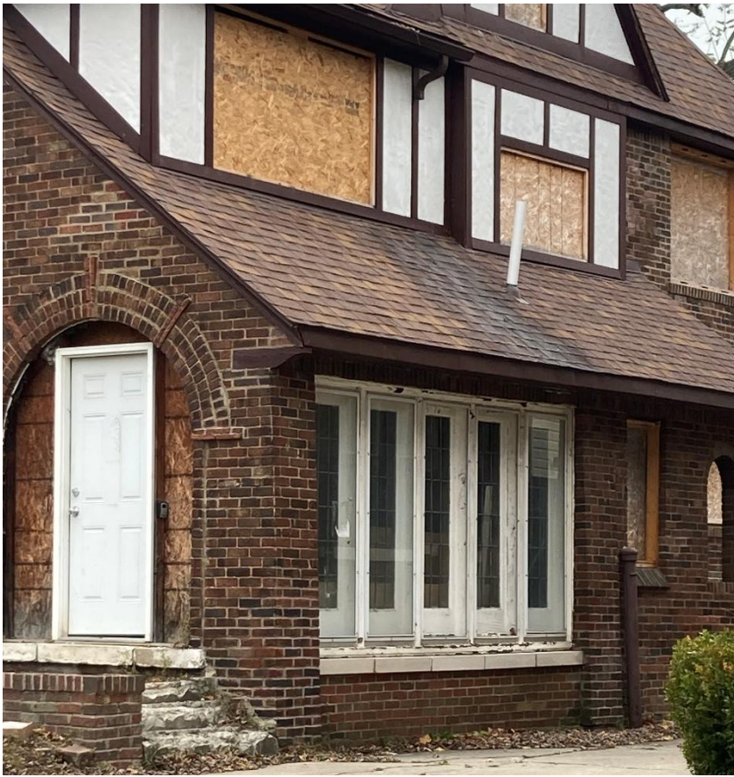
Current conditions. East wall showing only remaining original windows (wood casement with leaded glass), located at first story. Staff photo taken 11/25/2024
