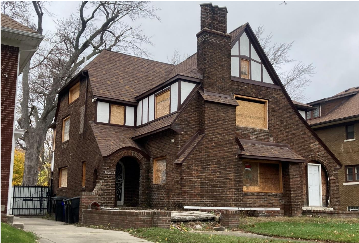
Current conditions. Note that the second and attic story have been rebuilt, most windows and associated casing/brickmould have been removed to the rough opening, and front door sidelites have been removed. Staff photo taken 11/25/2024
