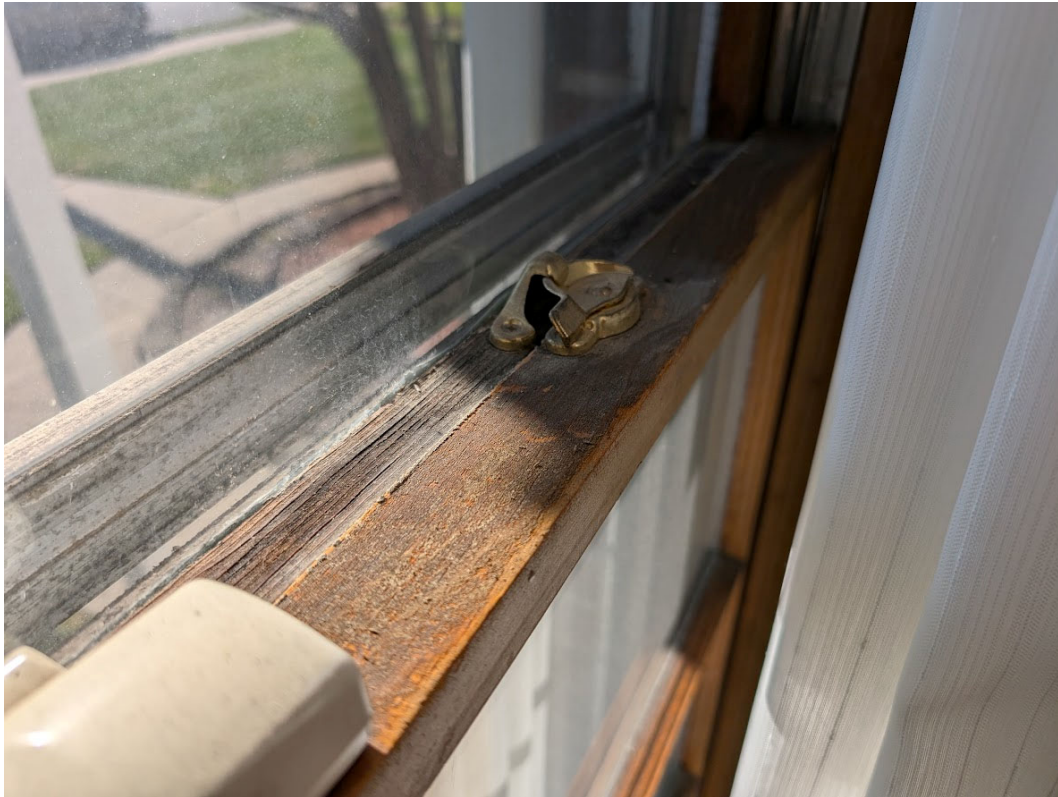
Detail view of a second floor, front window showing some visible deterioration at meeting rail. Staff photo, November 8, 2024.
