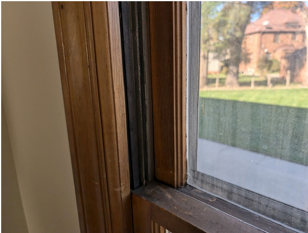
Detail view of window showing unitized nature (note aluminum channels). These windows are much tighter and stiffer than comparable pre-war wooden windows, and do not operate well. Staff photo, November 8, 2024.
