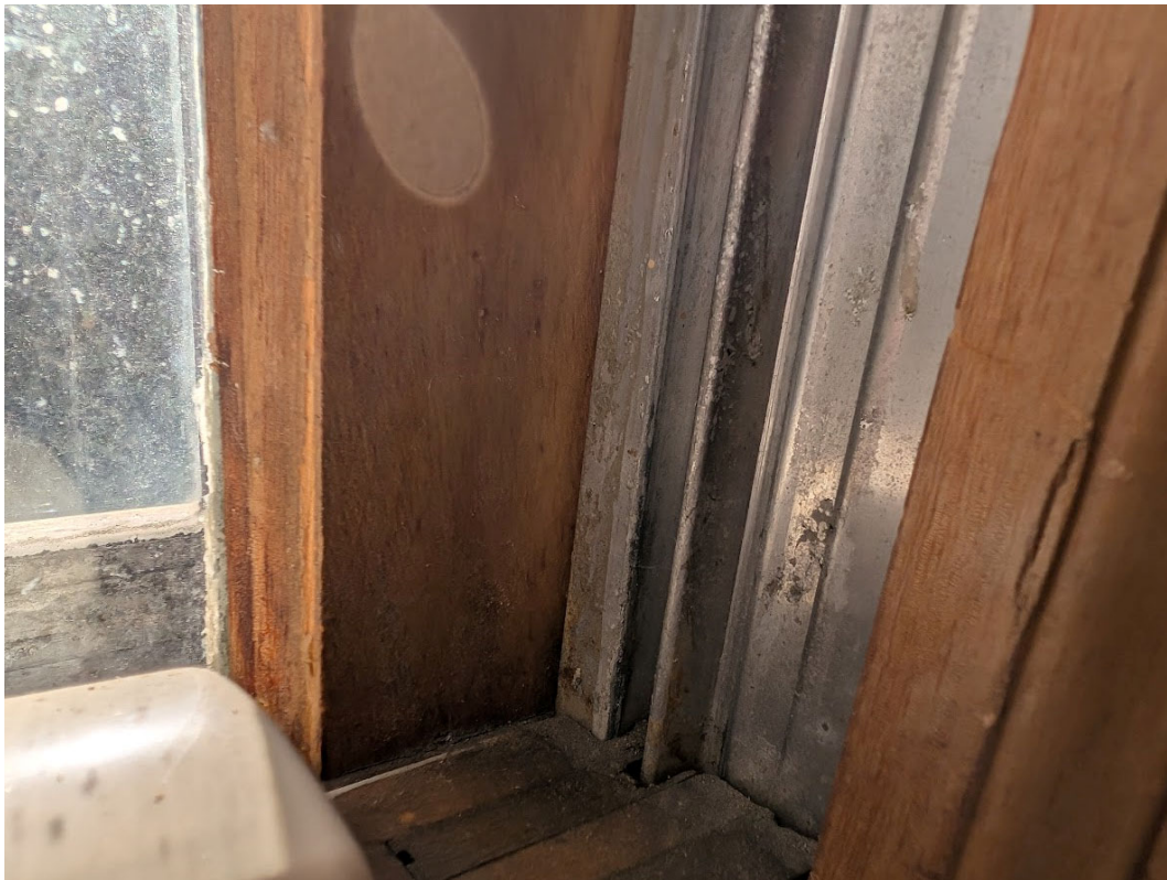
Detail view of another window showing incorporated sliding surfaces (aluminum channels) on which the unitized operation depends. Staff photo, November 8, 2024.
