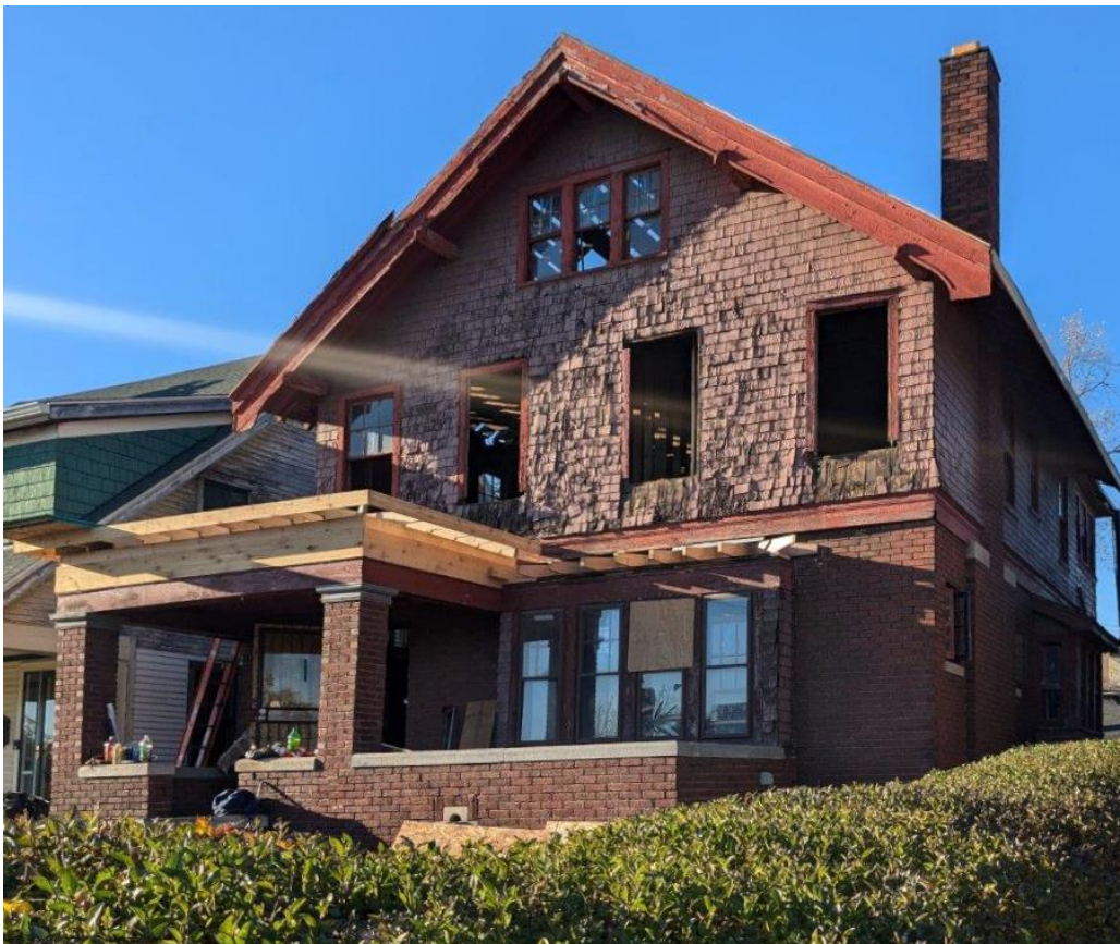
November 7, 2023 photo by staff. Fascia board on east elevation (upper right of image) added pursuant to November 1, 2024, Certificate of Appropriateness. New work visible above front porch (left side of image) was performed without approval and observed by staff November 7, 2024.
