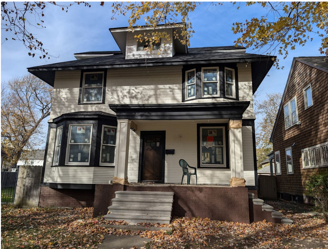
View of 708 Pallister, looking north from the sidewalk. Stop work order (orange sticker) is visible on one of the replaced windows. Staff photo, November 13, 2024.
