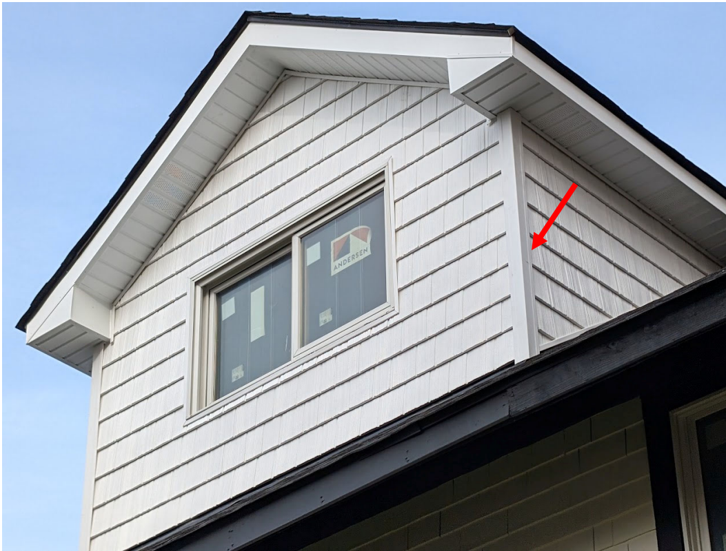
View of 708 Pallister, detail view of newly built west-facing (side) dormer. Note amateurish detailing, artificial shakes with imitation "wood grain" enclosed by corner trim pieces (red arrow), sliding vinyl-clad window, and vinyl clad eaves. Fascia boards also appear to be composite or vinyl rather than wood. Staff photo, November 13, 2024.
