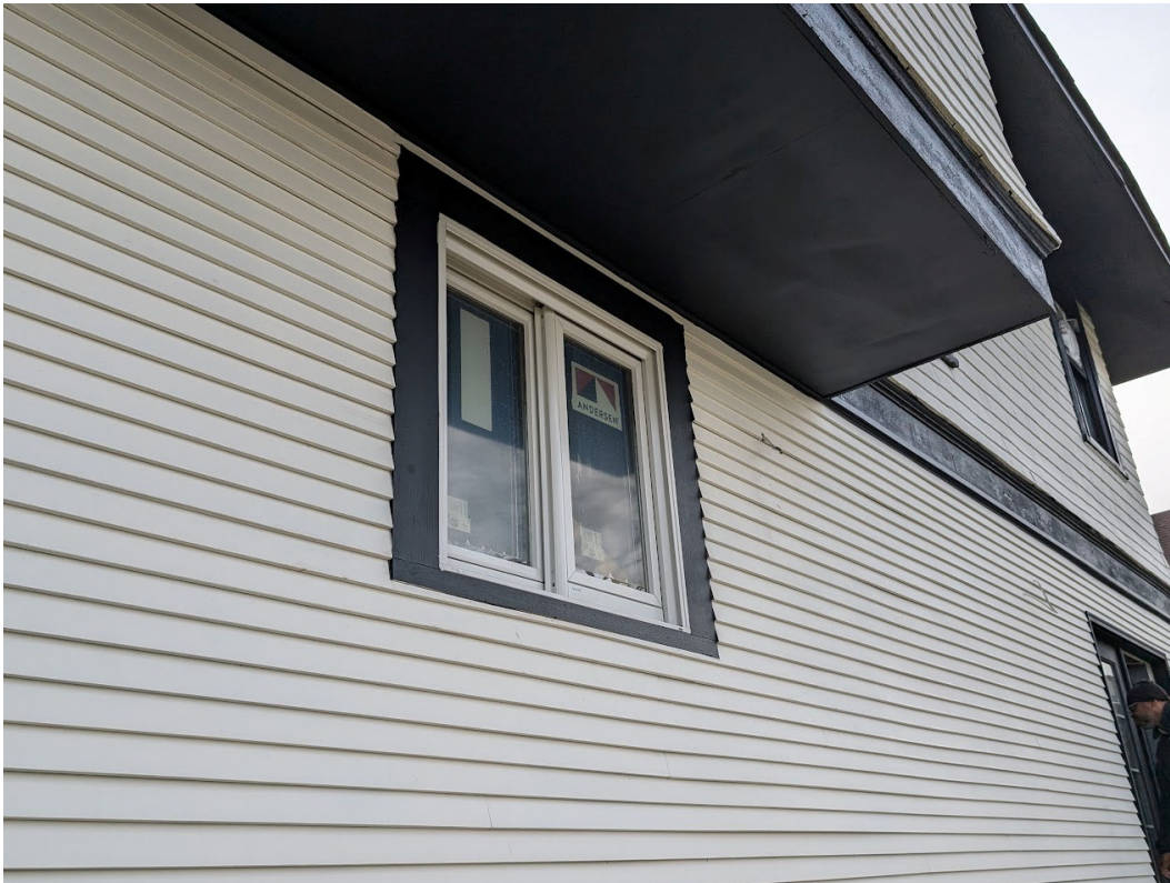
View of 708 Pallister, detail view of incorrect rear sliding window. Note also how the framing is recessed short of the clapboard surrounding it, an incorrect condition. Staff photo, November 13, 2024.
