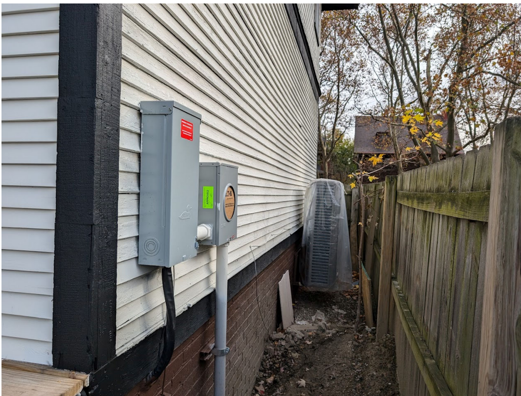
View of large HVAC unit under installation at west (side) wall. Staff photo, November 13, 2024.
