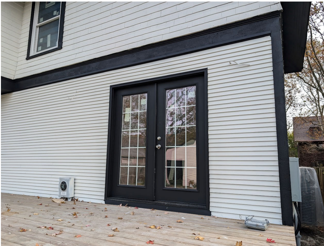
Rear view of 708 Pallister, detail view of incorrect French doors with internal imitation muntins, contrary to the Commission's conditional approval of custom reproduction 2/1 units. Staff photo, November 13, 2024.
