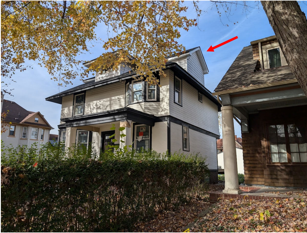
View of 708 Pallister, looking northwest from the sidewalk. Note large east-facing dormer at right side, with incompatible gable roof and no window at all. Staff photo, November 13, 2024.
