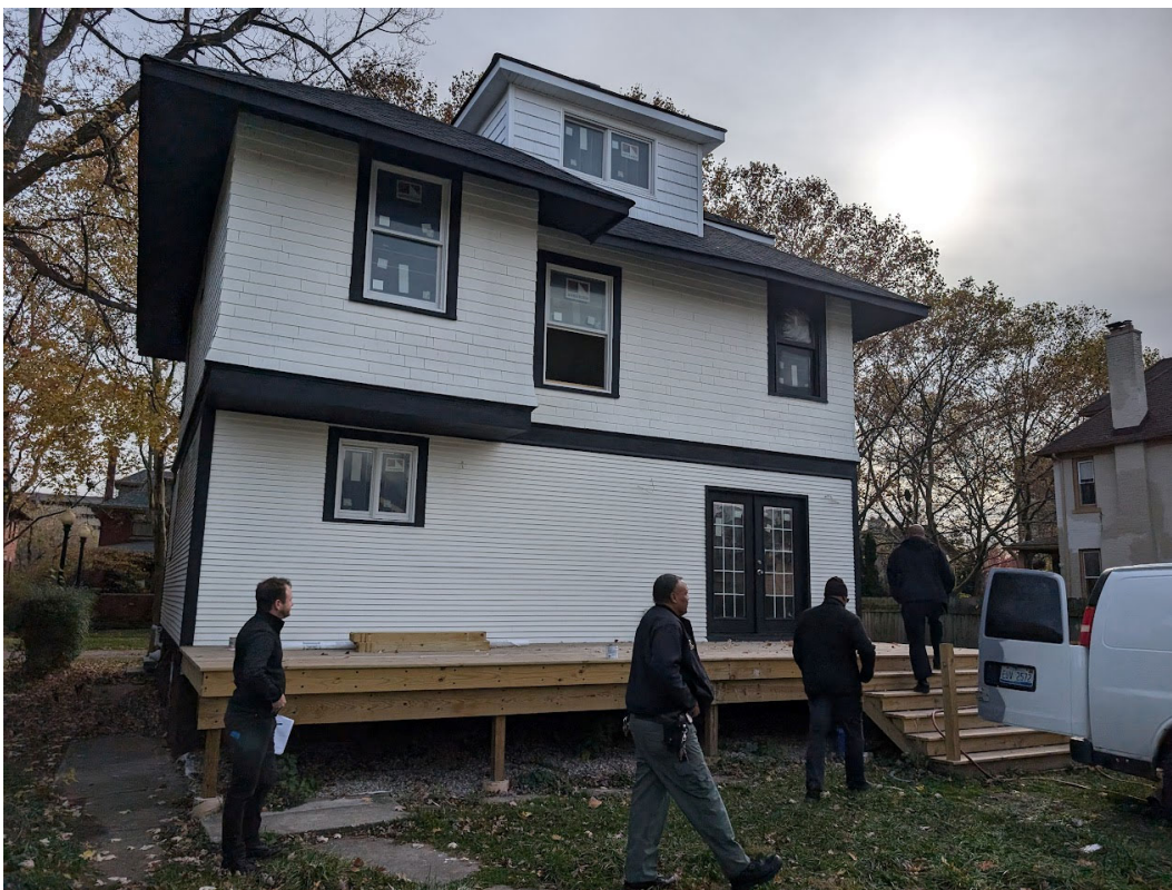
View of 708 Pallister, at the rear. Visible are the incorrect eastward sliding window (left), and the incorrect French doors with "between-the-glass" grids, right. Note also the factory white roof dormer, incorrectly clad with imitation shake and with a sliding window installed, as compared to the "yellowish white" of the approved HDC color choice. Building inspectors and NPO are visible here. Staff photo, November 13, 2024.
