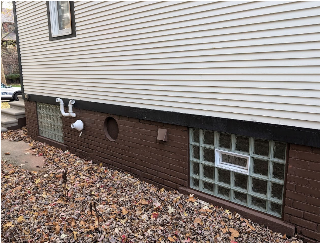
View of glass block windows at east side basement wall. Staff photo, November 13, 2024.
