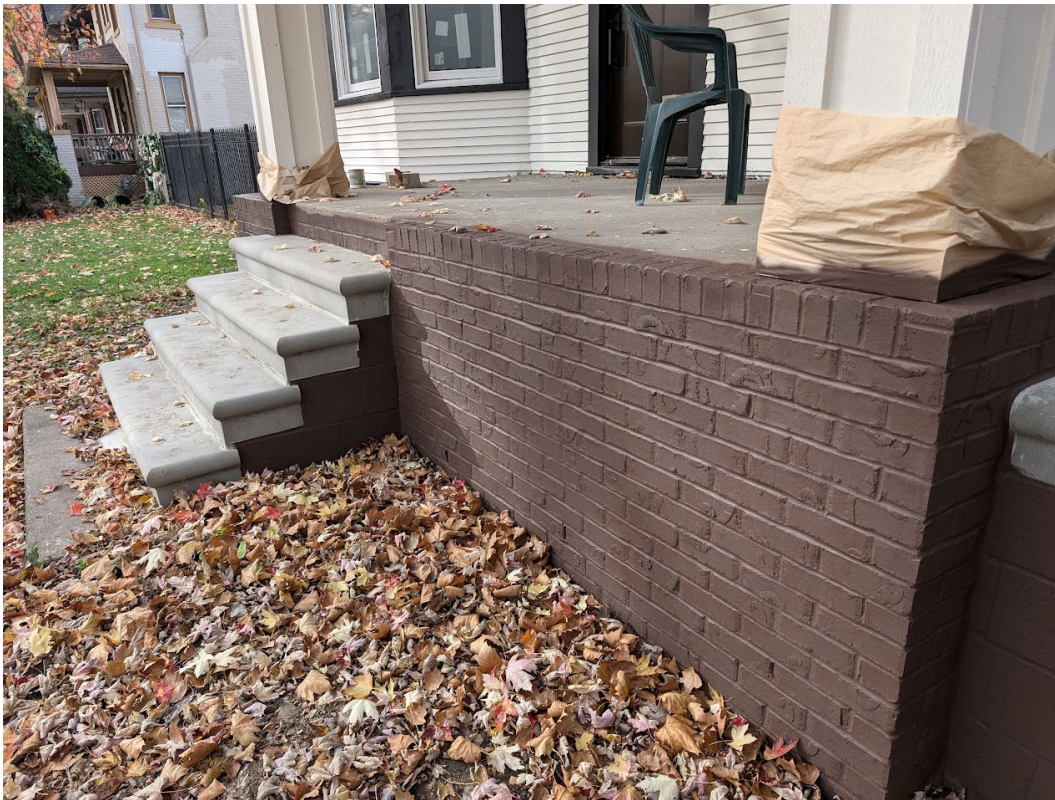
Newly painted brick veneer and steps at front porch. Staff photo, November 13, 2024.
