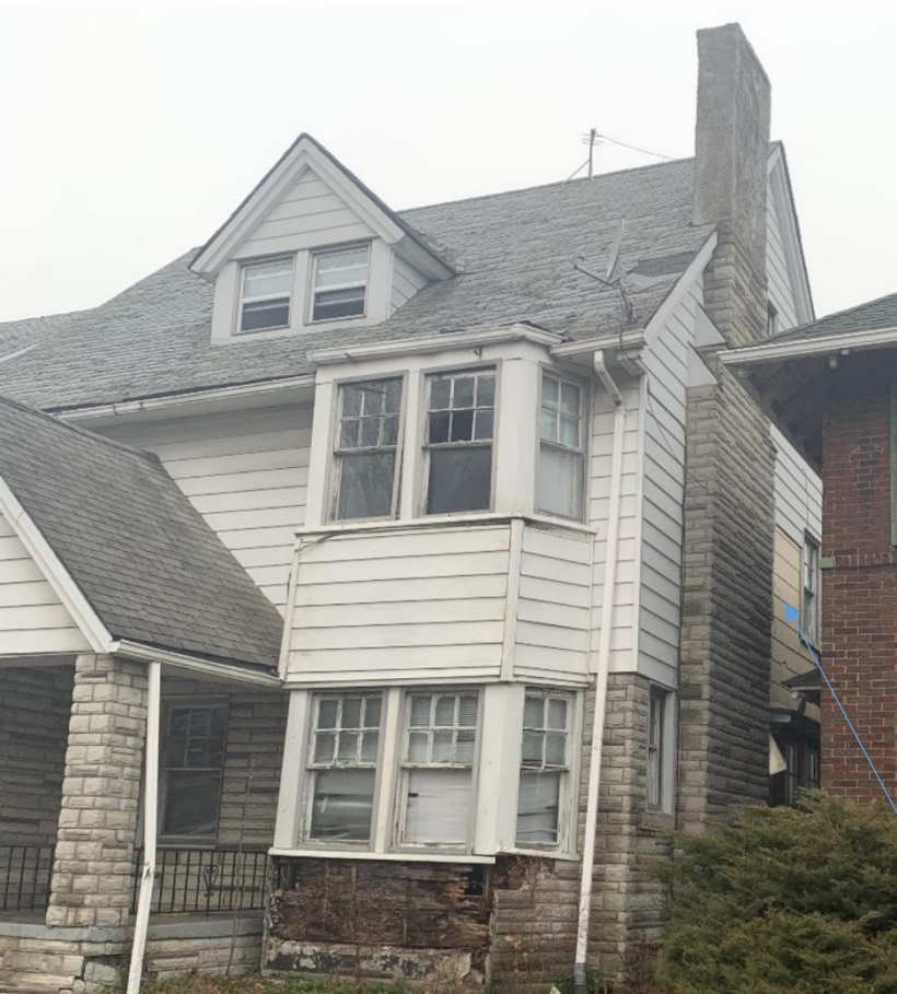
Photo taken in 2020 by previous applicant. Note area where aluminum siding has fallen off, revealing synthetic shingle siding underneath.
