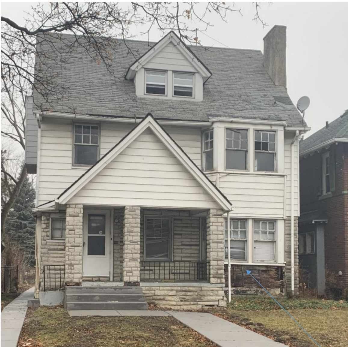
Front façade, 2020 photo taken by previous applicant. Note area where Permastone has fallen off
