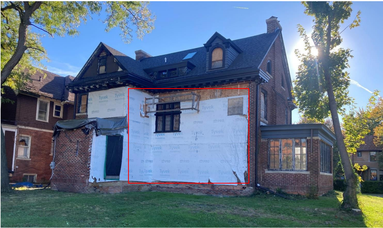
Current condition at rear wall, staff photo taken on 10/16/2024. Area outlined in red indicates proposed location for lapped wood siding.
