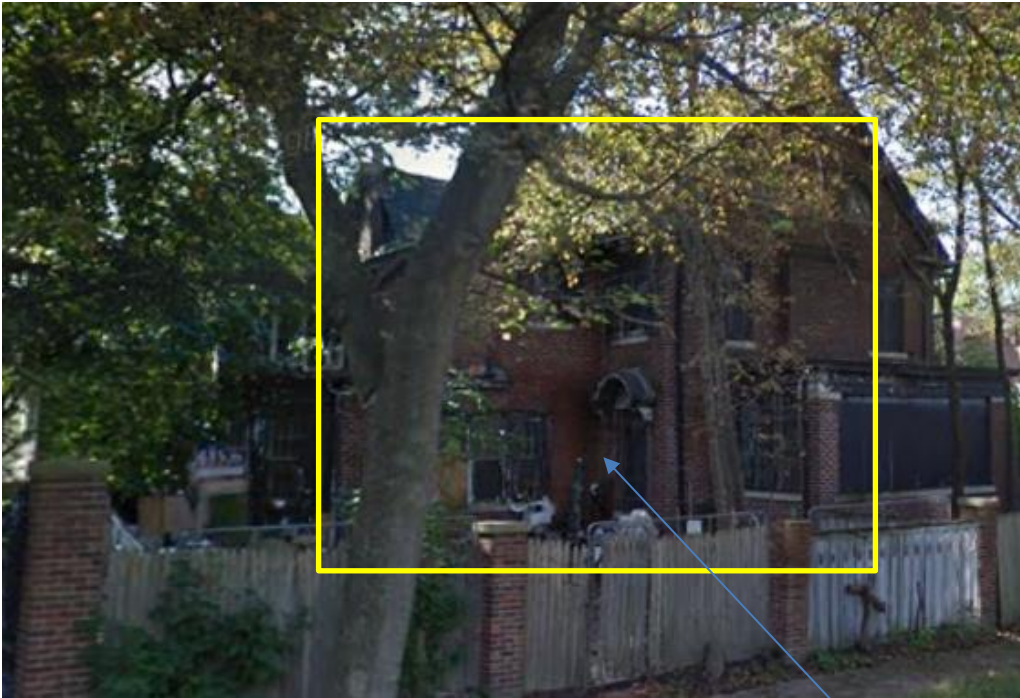
Google Streetview image of the rear dating from 2011. Note that the area outlined in yellow shows the rear two-story addition which had collapsed by 2019. Specifically see where the south wall of the addition is located in relation to the door and canopy at the rear.
