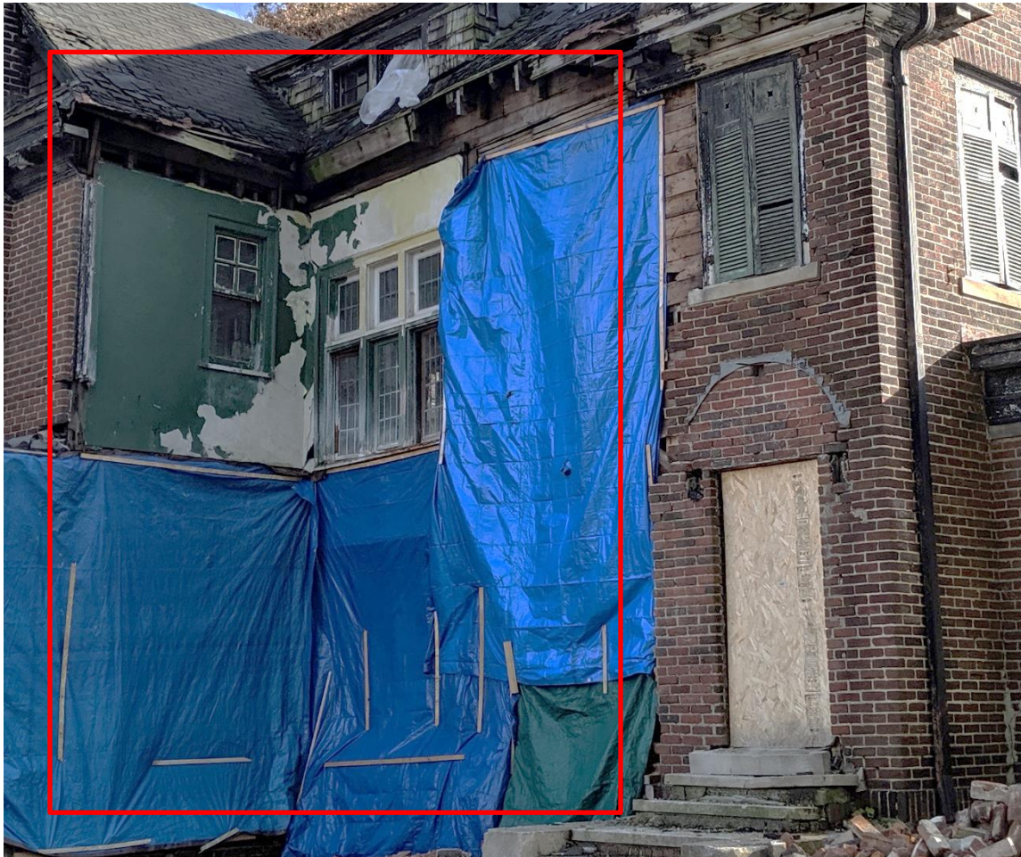
Staff photo of the rear dating from 2019. Note that the two-story addition is no longer present/had collapsed ca. ca. 2018, leaving the plaster which covered former interior wall exposed (outlined in red).
