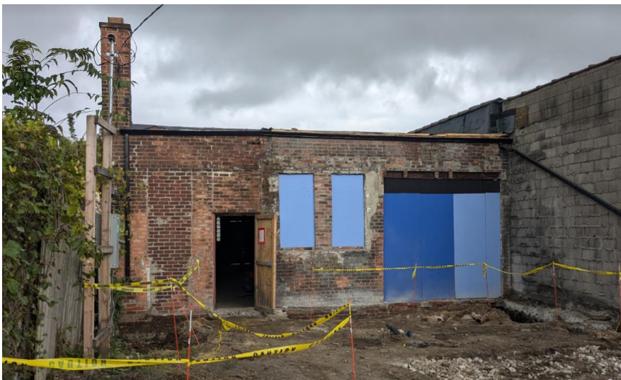
Rear (south) of building viewed from the alley. October 2024 photo by staff.
