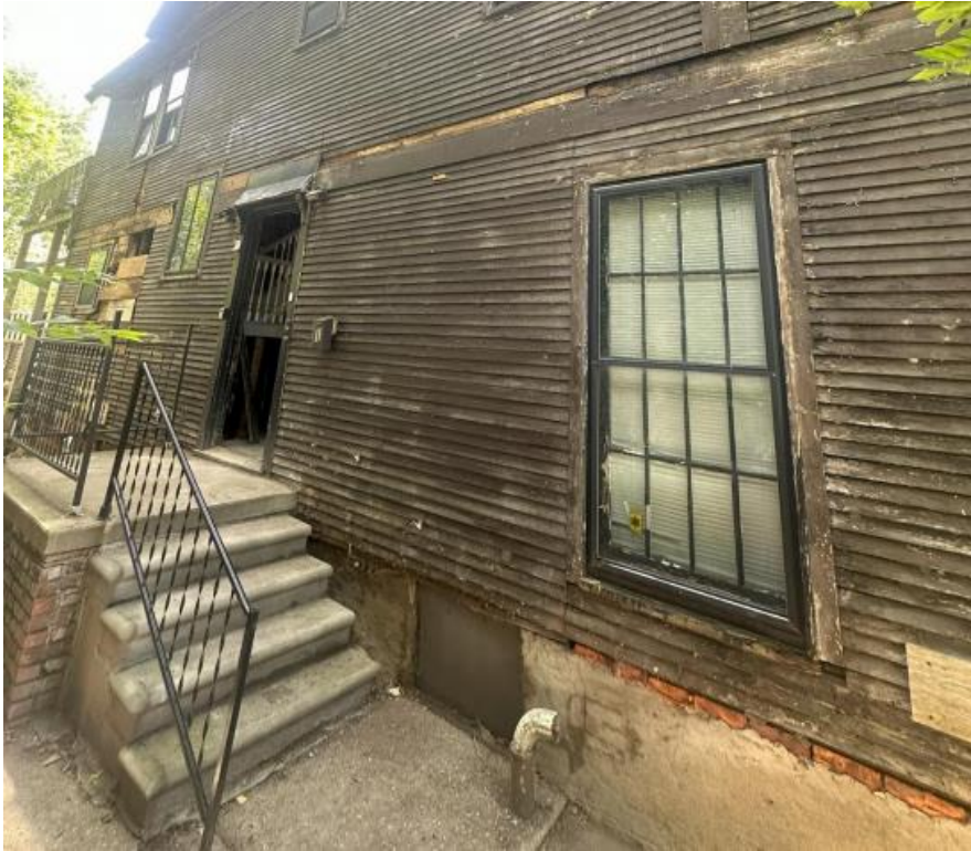
7873 Van Dyke Place, west/side wall. Location of current primary entry door. Photo taken by staff on 8/30/2024
