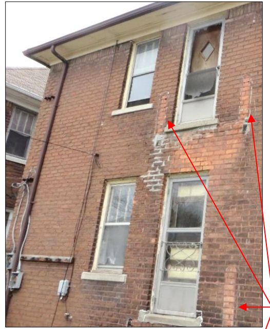
2018 photo of rear elevation. "Ghost" images of the original porch are evident on the brick.
