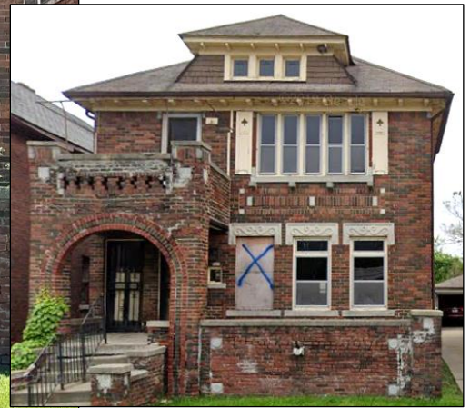
Below: The 2019 Google street view image shows the wood bracketed soffit and wood fascia still intact.
