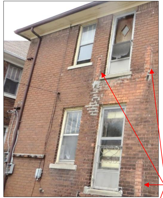
2018 photo of rear elevation. "Ghost" images of the original porch are evident on the brick.
