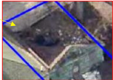
This close-up view appears to show the back/alley-facing wall had fallen inward.
