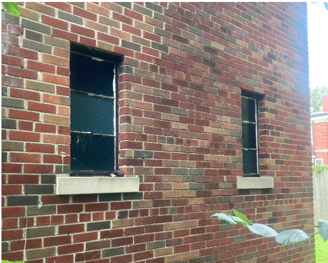
These 2 windows at the rear/southwest corner of the building’s sanctuary are proposed for replacement with aluminum-clad wood casement units. Staff photo taken 9/6/2024
