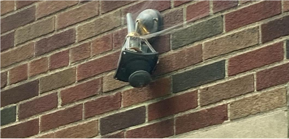
1818 Seminole. Facing light at east wall of the rear flat roof wing which is proposed for replacement. Staff photo taken on 9/6/2024
