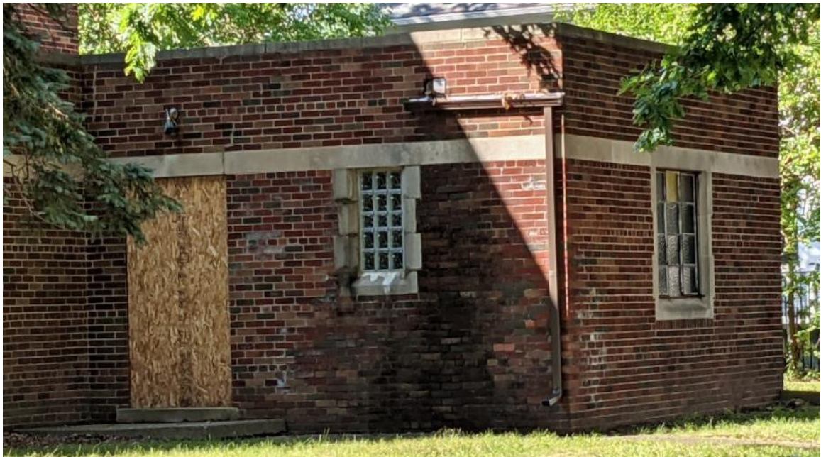
Front and side wall of rear, flat roof wing. Note decorative stone surrounds and stone course above door and window openings. Staff photo taken 9/6/2024
