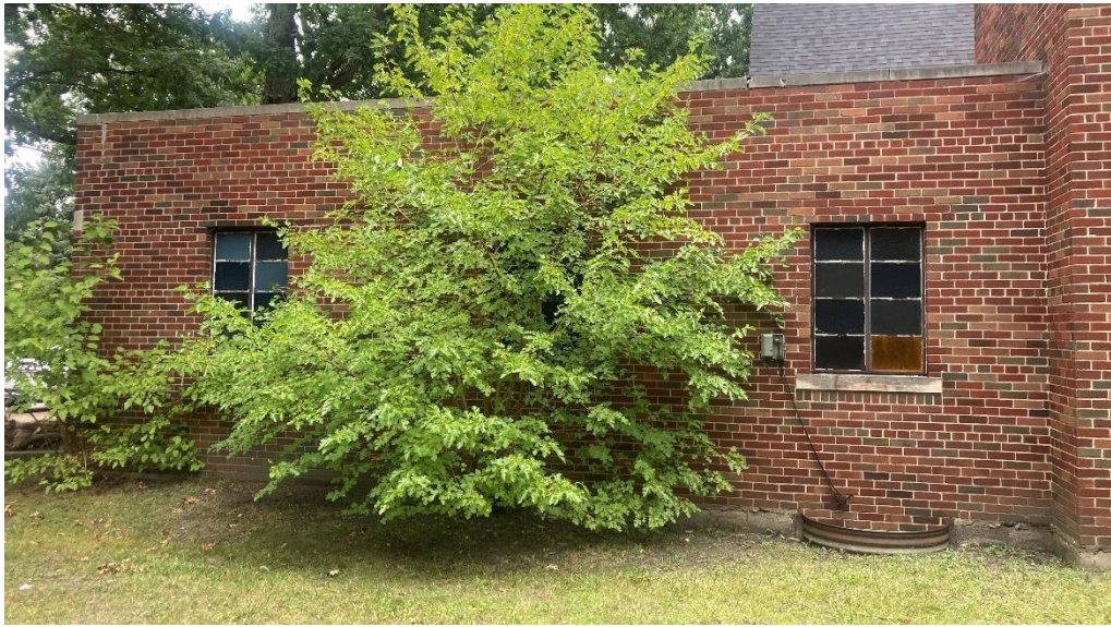
Rear wall of flat-roof wing proposed for removal in order to accommodate new garage extension. Note lack of detailing at window surrounds and wall.
