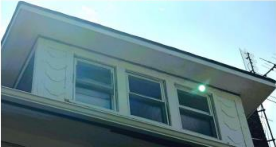
Front dormer. Note that front wall is clad with a scalloped wood siding while sidewalls are covered with asphalt shingles. Photos provided by applicant.
