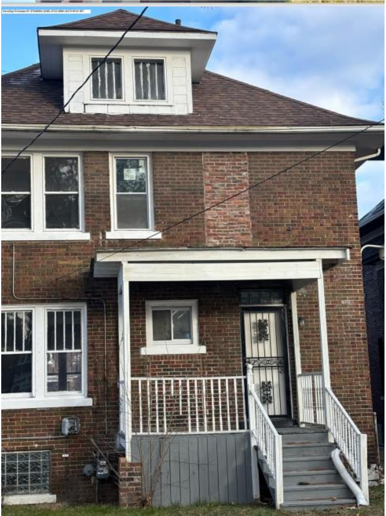
Rear wall, showing 4/1 double hung wood windows and 4-lite wood casement windows prior to current unapproved work. Note that the 1/1 vinyl windows at the second story and the small slider window at the first story are also recent unapproved alterations likely added prior to the current applicant's ownership. Photo provided by applicant.
