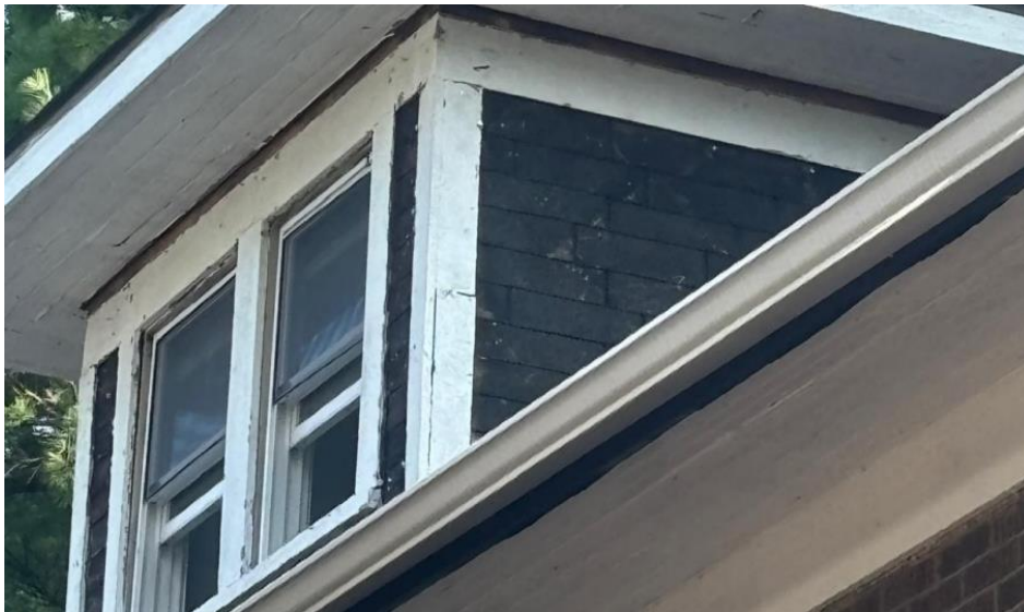
The two dormers at the side walls are clad with asphalt shingles. Photo provided by applicant.
