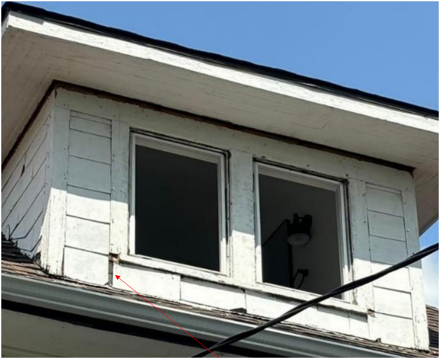
Rear dormer. Note that front wall is clad with wood siding while sidewalls are covered with painted asphalt shingles. Asphalt shingle is visible below wood siding at this location. Photos provided by applicant.
