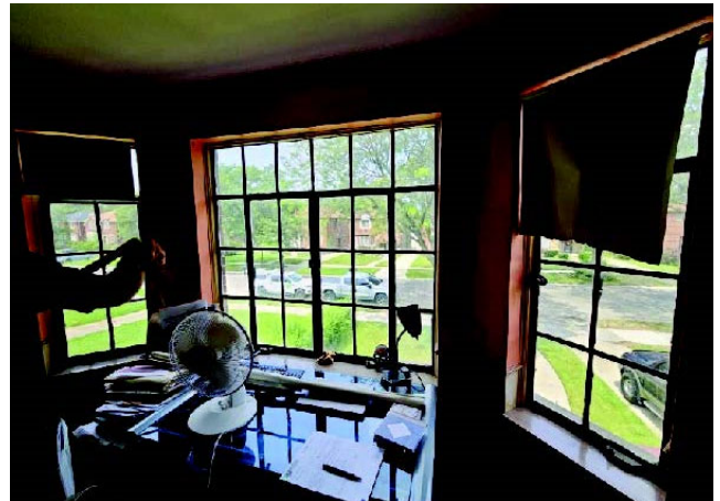
Figure 6, by Applicant: Windows 202-204, (North Interior, 2 nd floor) Interior casements proposed to be replaced with fibrex windows.
