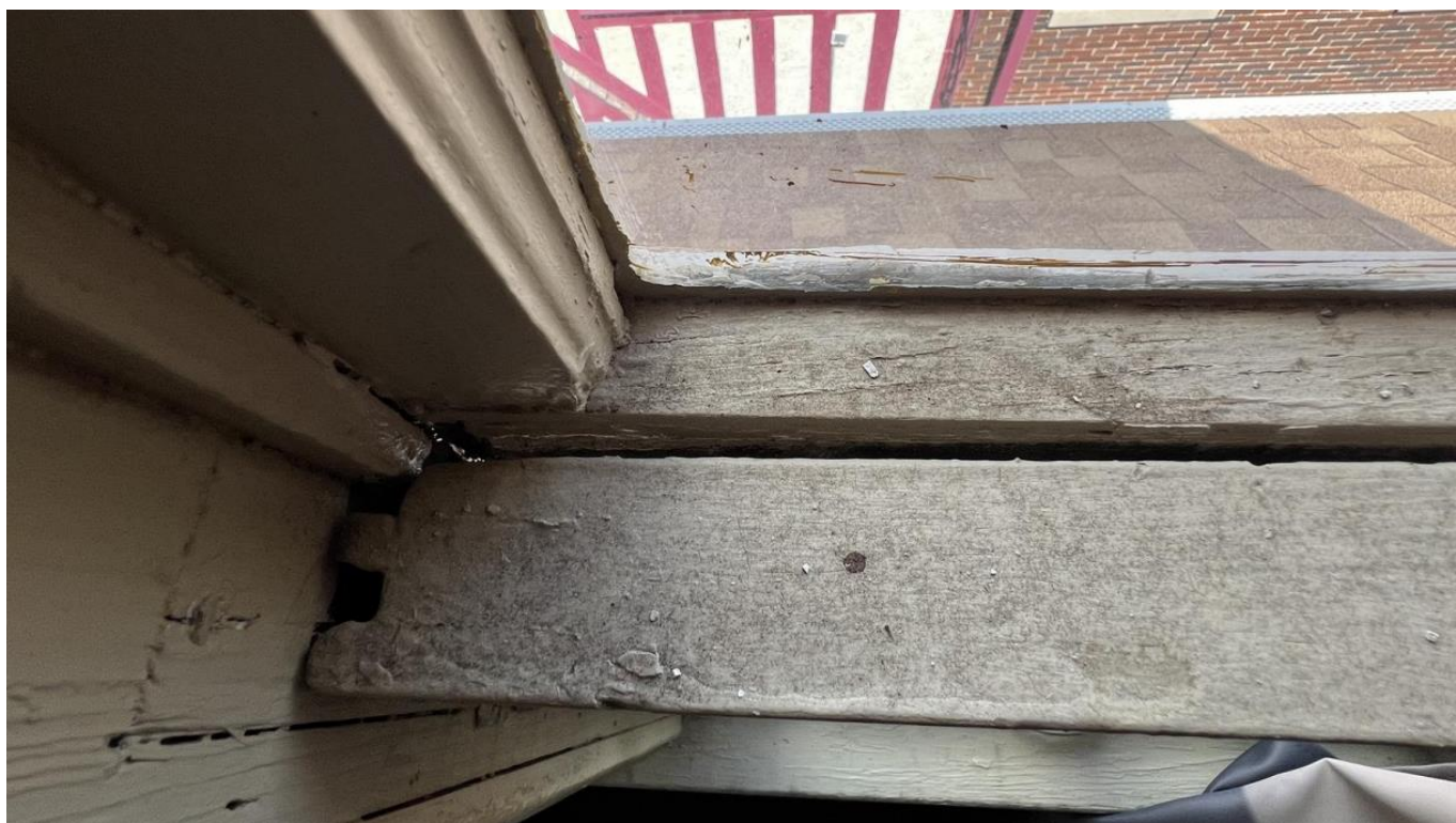
Photo from application showing peeling paint and missing sash cord.
