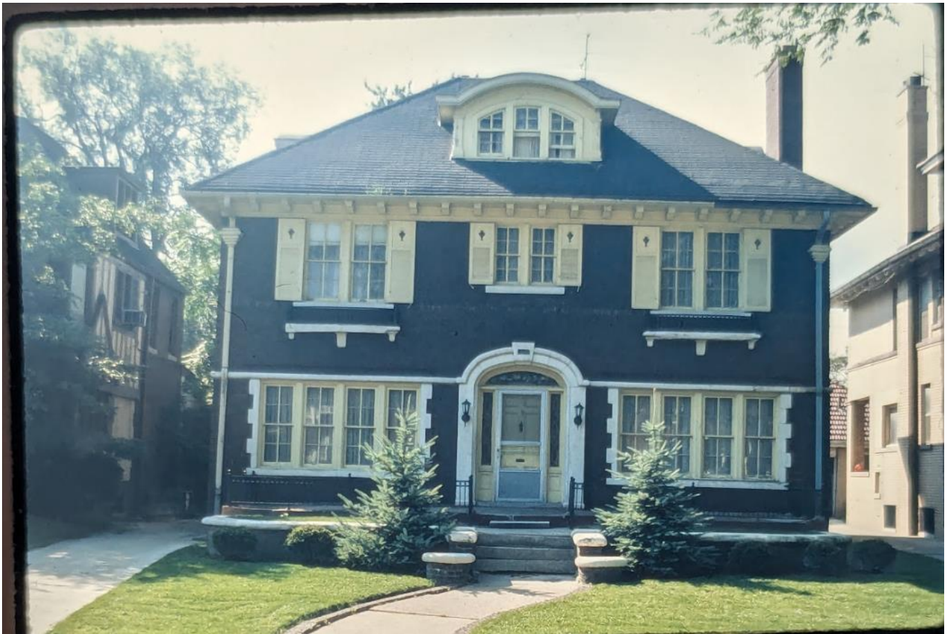
1974 photo by the Historic Designation Advisory Board. Note character-defining four-over-four windows since replaced without approval.
