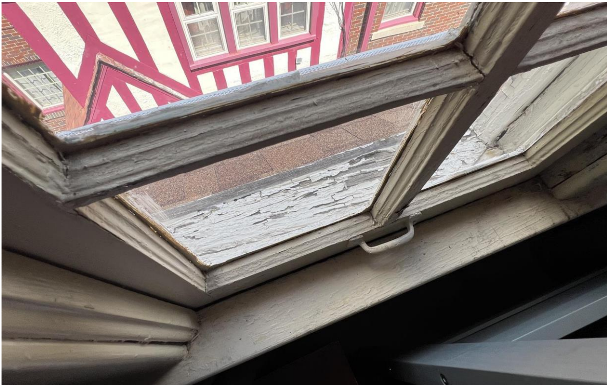
Photo from application showing peeling paint.
