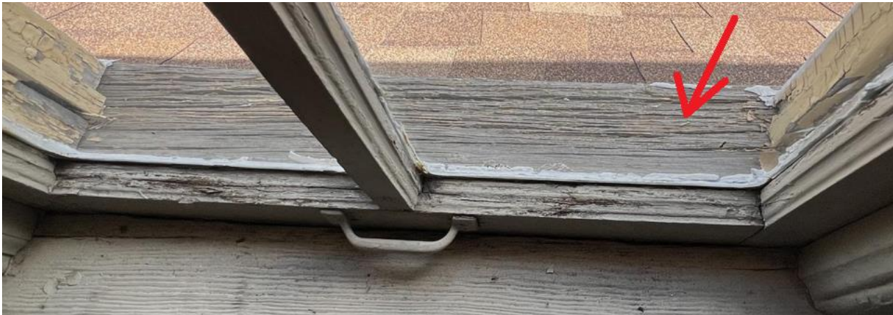
Application photo showing deterioration of sill; cropped by staff with arrow added.
