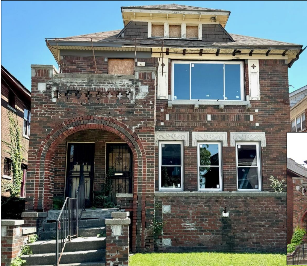
Left: Staff photo, July 26, 2024. This condition of the soffit and fascia has been in place since at least September 2021 when staff first photographed this property.
