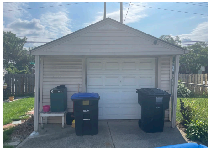
Site Photo 2, by Staff July 25, 2024: (West) front elevation of the existing garage.
