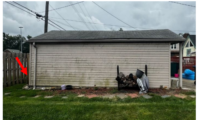
Site Photo 5, by Applicant, showing north side of the existing garage. The arrow indicates the location of past vehicle impact.
