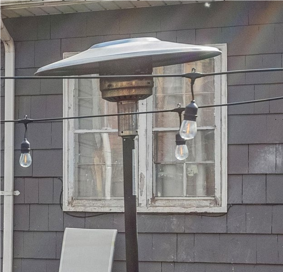
Figure 10: Original, paired, four-over-four windows with wood storms present at the rear of the property.
