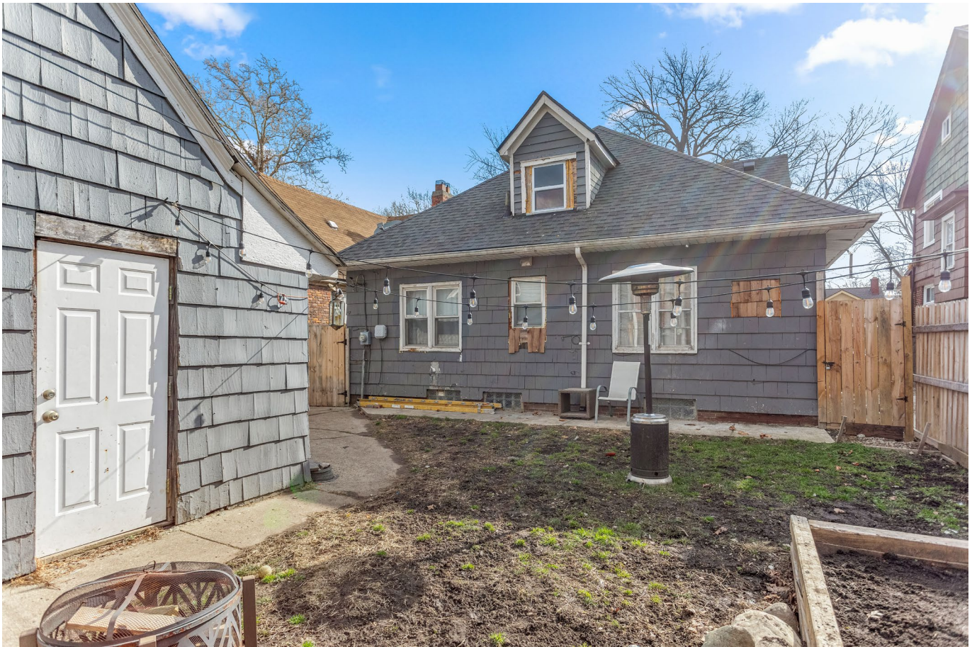
Figure 4: Image showing rear of dwelling with new windows and an infilled window opening. A replacement pedestrian door at the garage is not included with this application.
