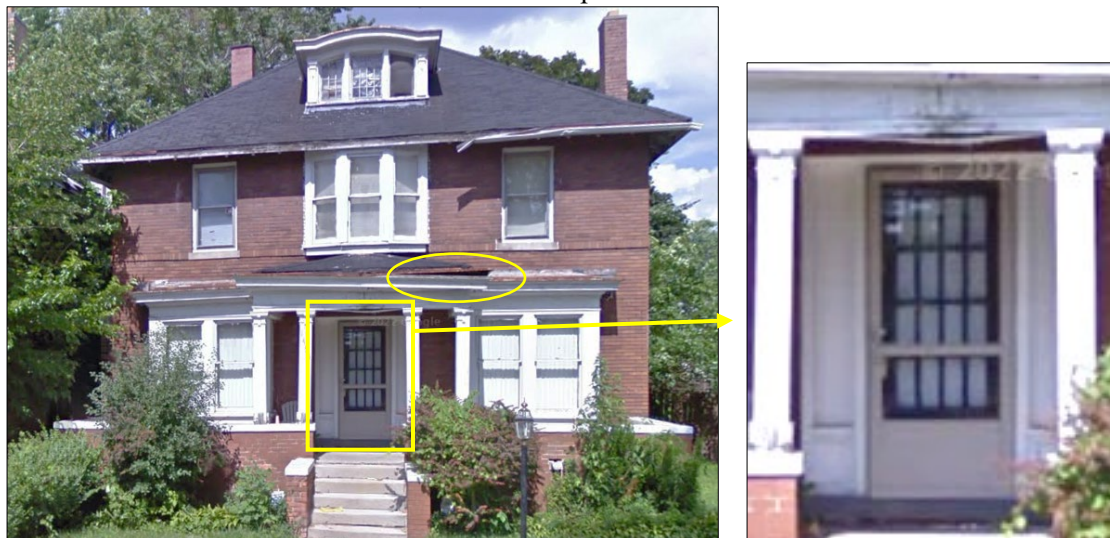
July 2009, Google streetview. The porch roof is beginning to sag, but otherwise the façade is intact. This photo offers a good view of the 16-light wood front door and wood side panels.
