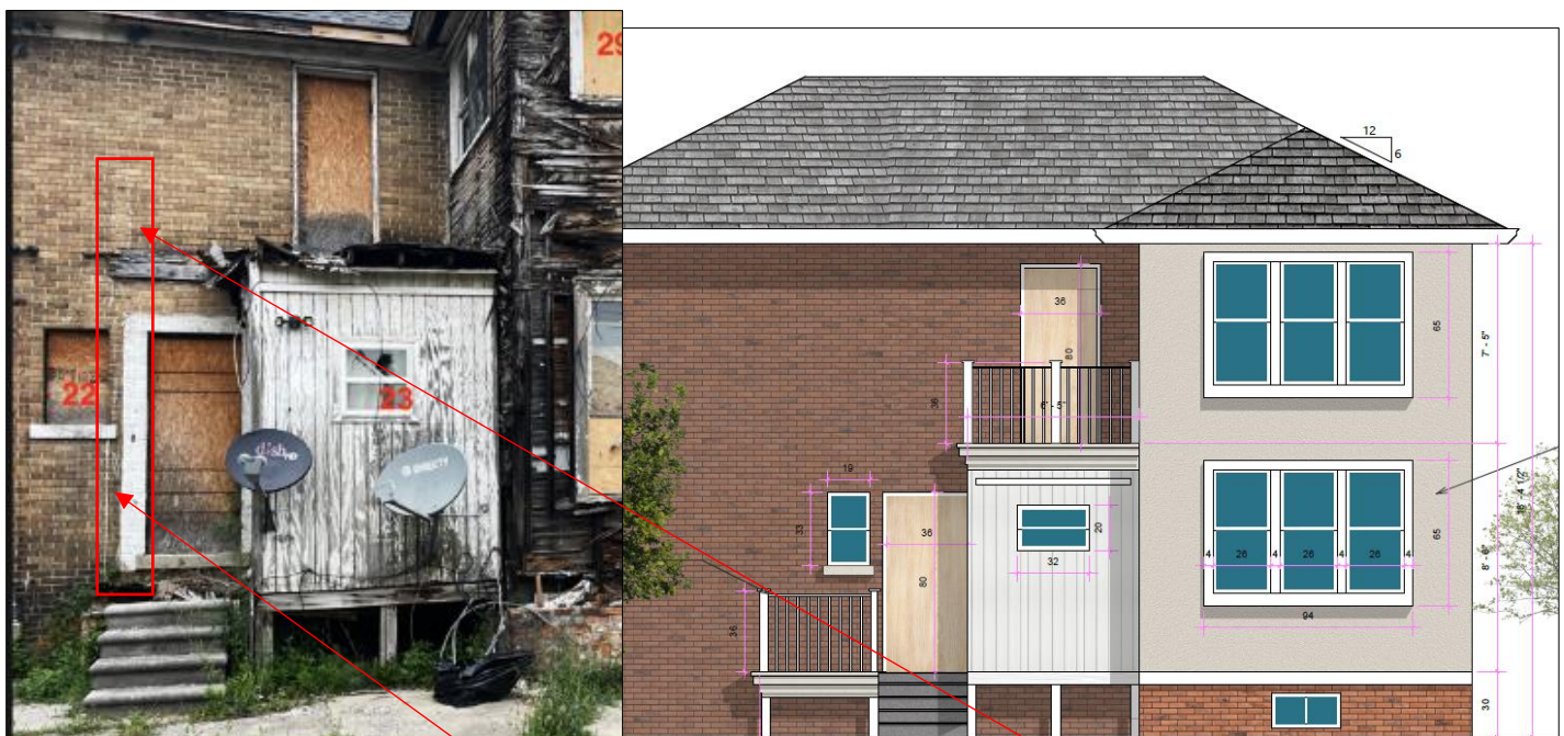
Applicant drawing. Remaining paint line adjacent first floor door opening and ghost image of upper porch railing offer evidence of the original two-story porch footprint (enclosure covered with T1-11 siding was originally part of the open porch).
