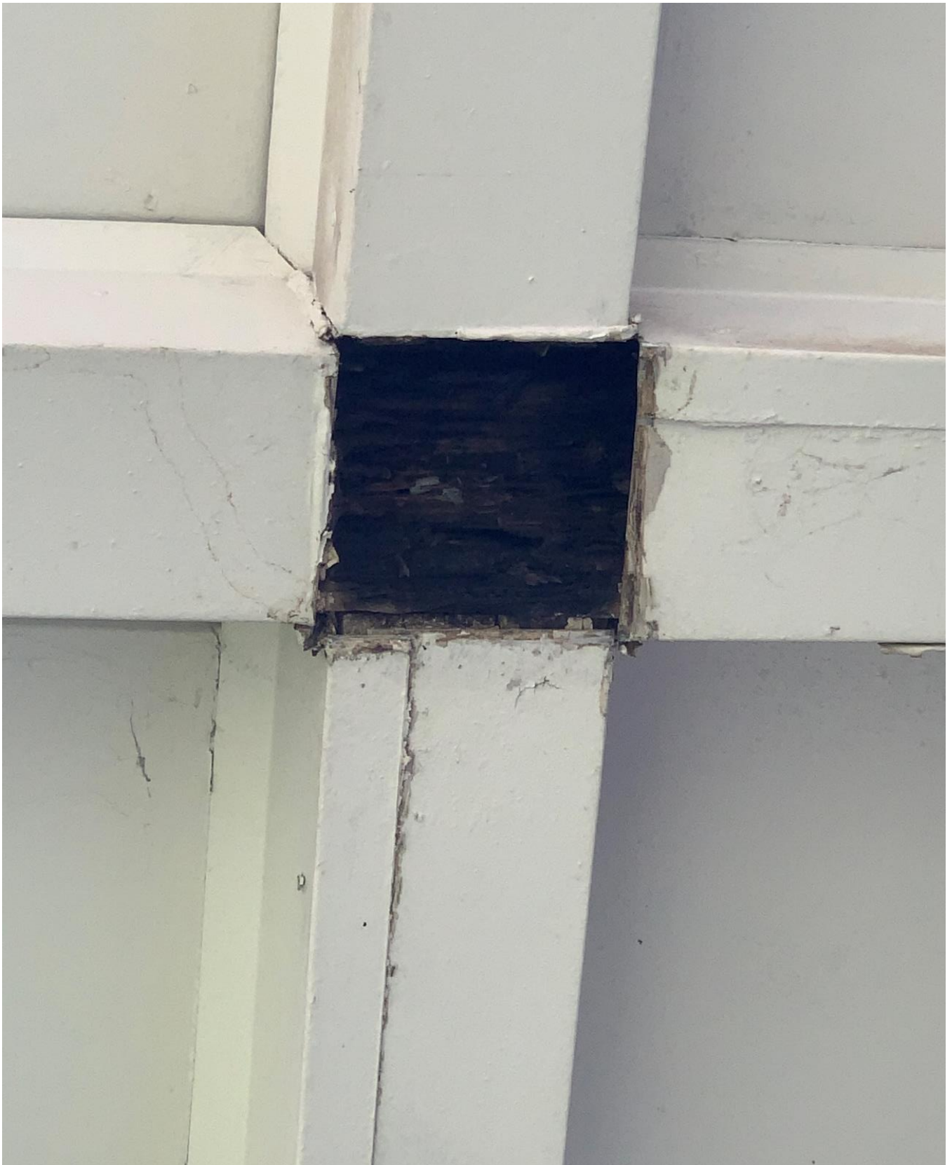
Photo by applicant. Detail of wood bracket in the eaves at the rear elevation. Showing area of wood rot.
