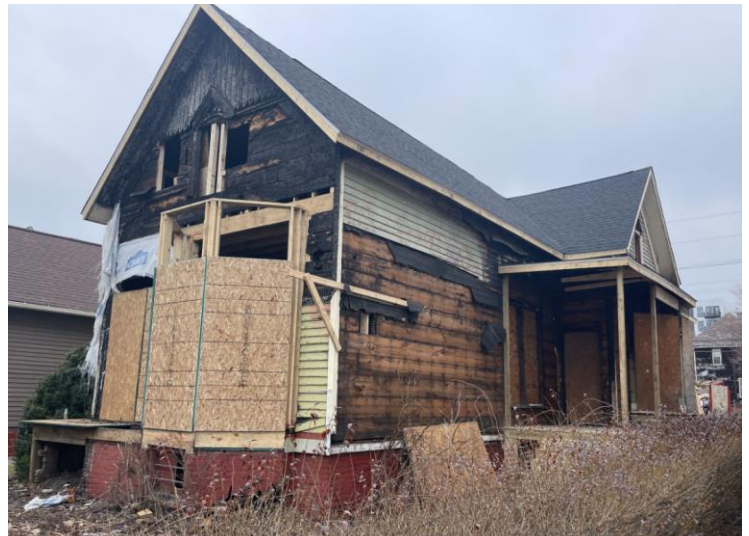
Appearance in 2/2024, after unapproved work. HDC staff
