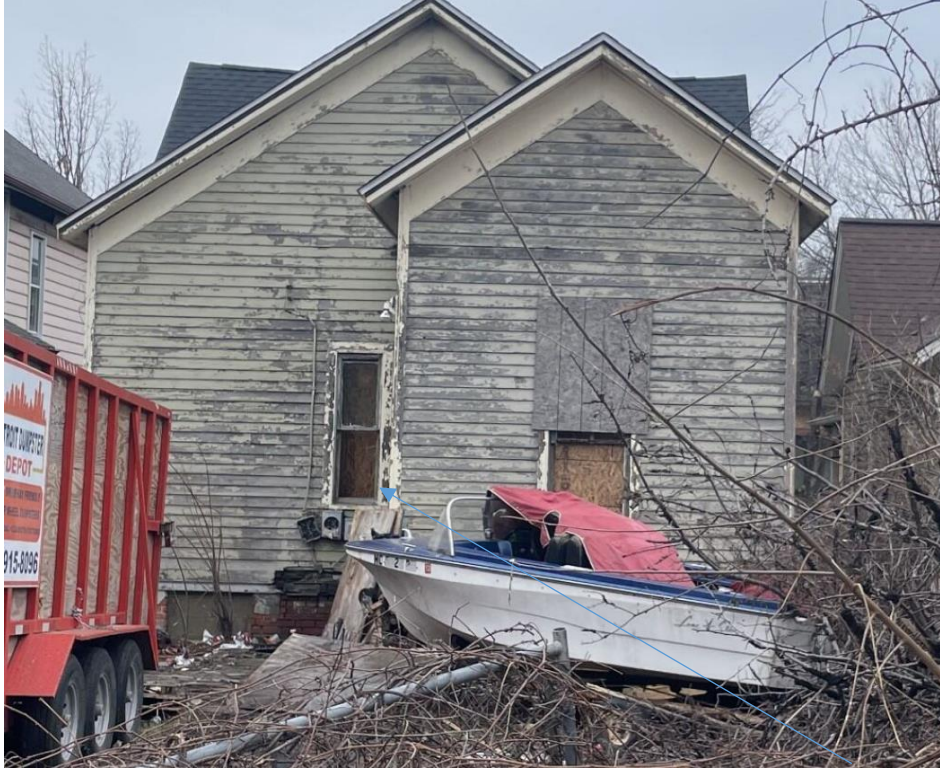
Rear, photo taken by HDC staff in 2/2024. Note that the window to the left was removed without HDC approval sometime between 2/2024 and 6/2024.
