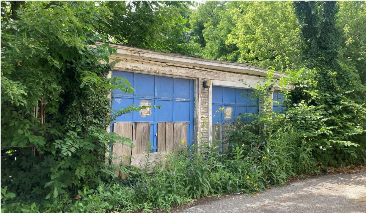
1108 Van Dyke garage, facing northwest showing current appearance of garage. Staff photo taken on 6/25/2024
