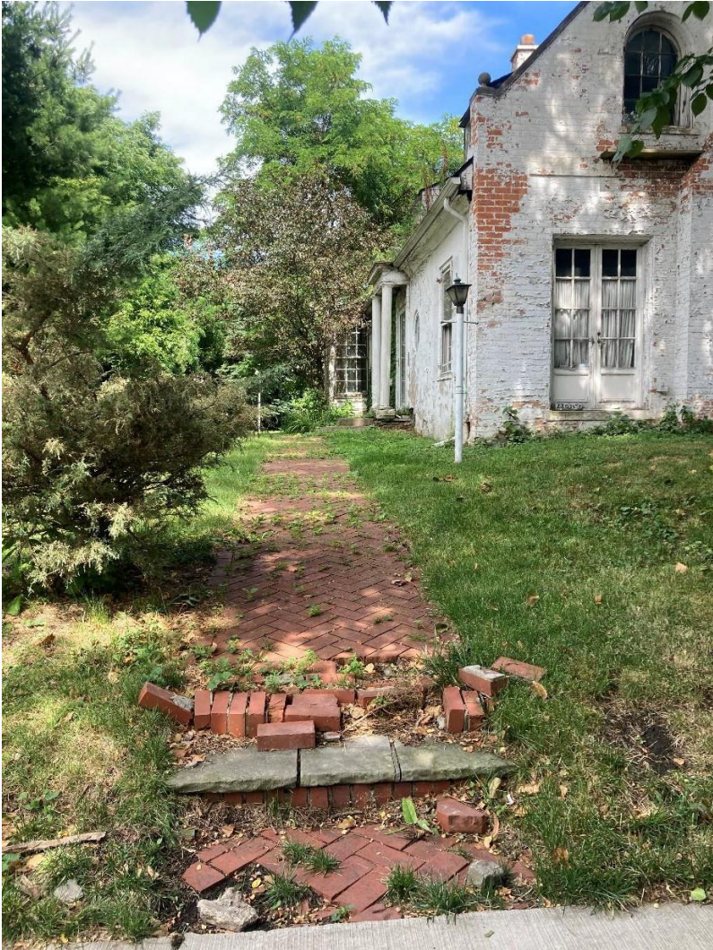
1108 Van Dyke, facing east showing brick walkway and steps with stone treads. Staff photo taken on 6/25/2024
