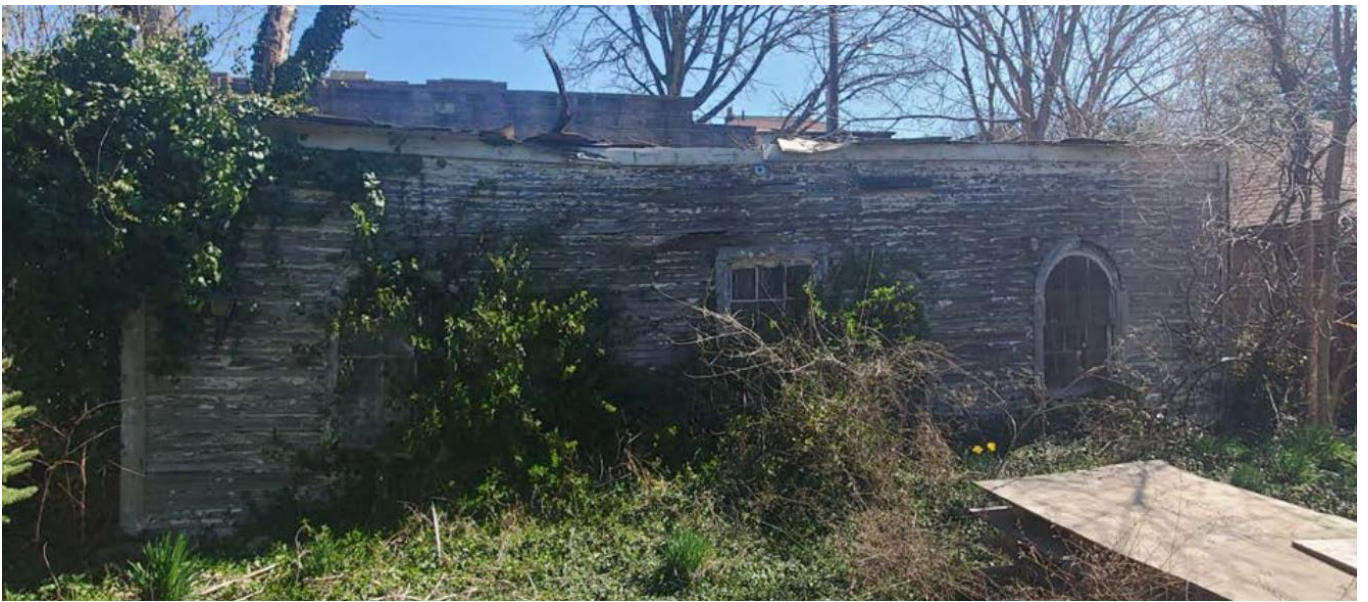
1108 Van Dyke garage, facing southeast showing current appearance. Photo provided by applicant
