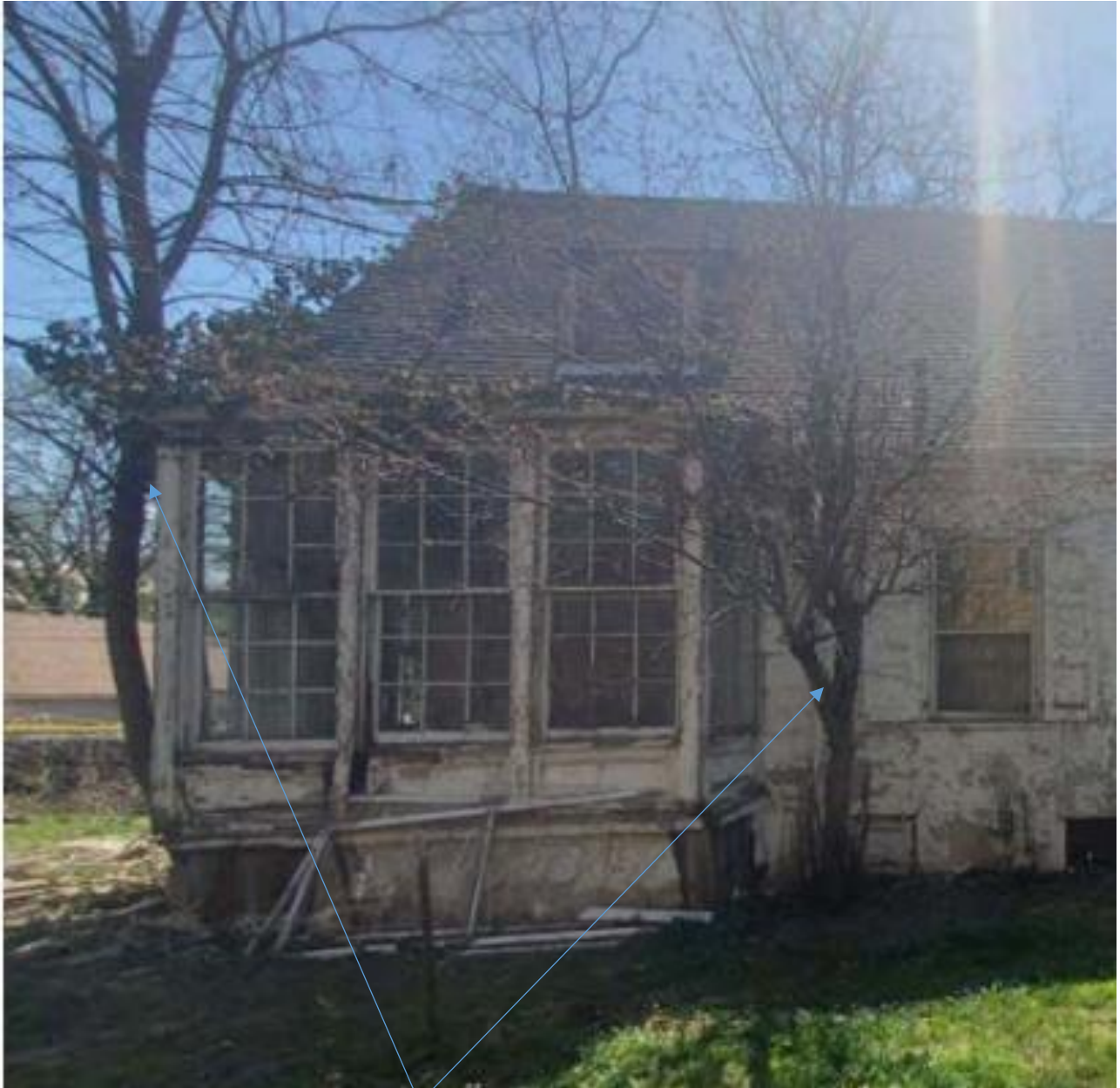
1108 Van Dyke, north bay. These two trees are proposed for removal due to their close proximity to the building's foundation and their potential to damage the foundation
