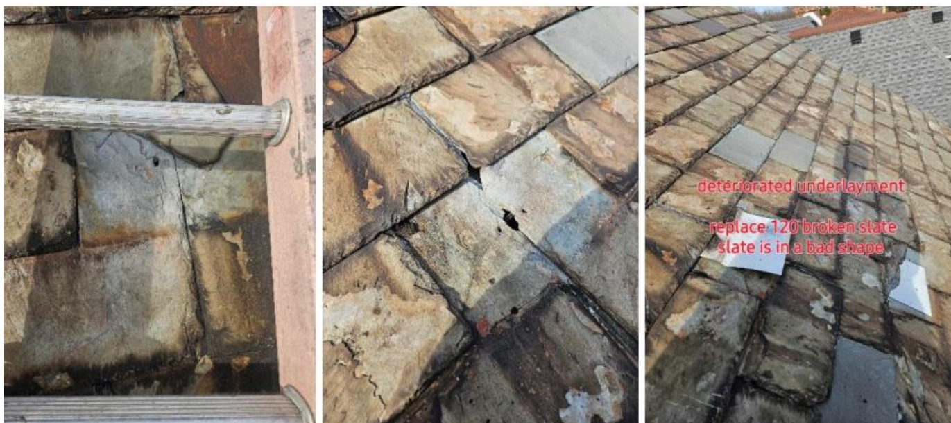
Photos provided by Detroit Cornice and Slate. Please see the application materials for additional photos and higher resolution.
