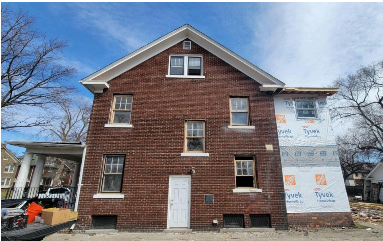
1485 Longfellow, current conditions. Facing south. Note new two-story addition which was erected without HDC approval. Photo provided by applicant
