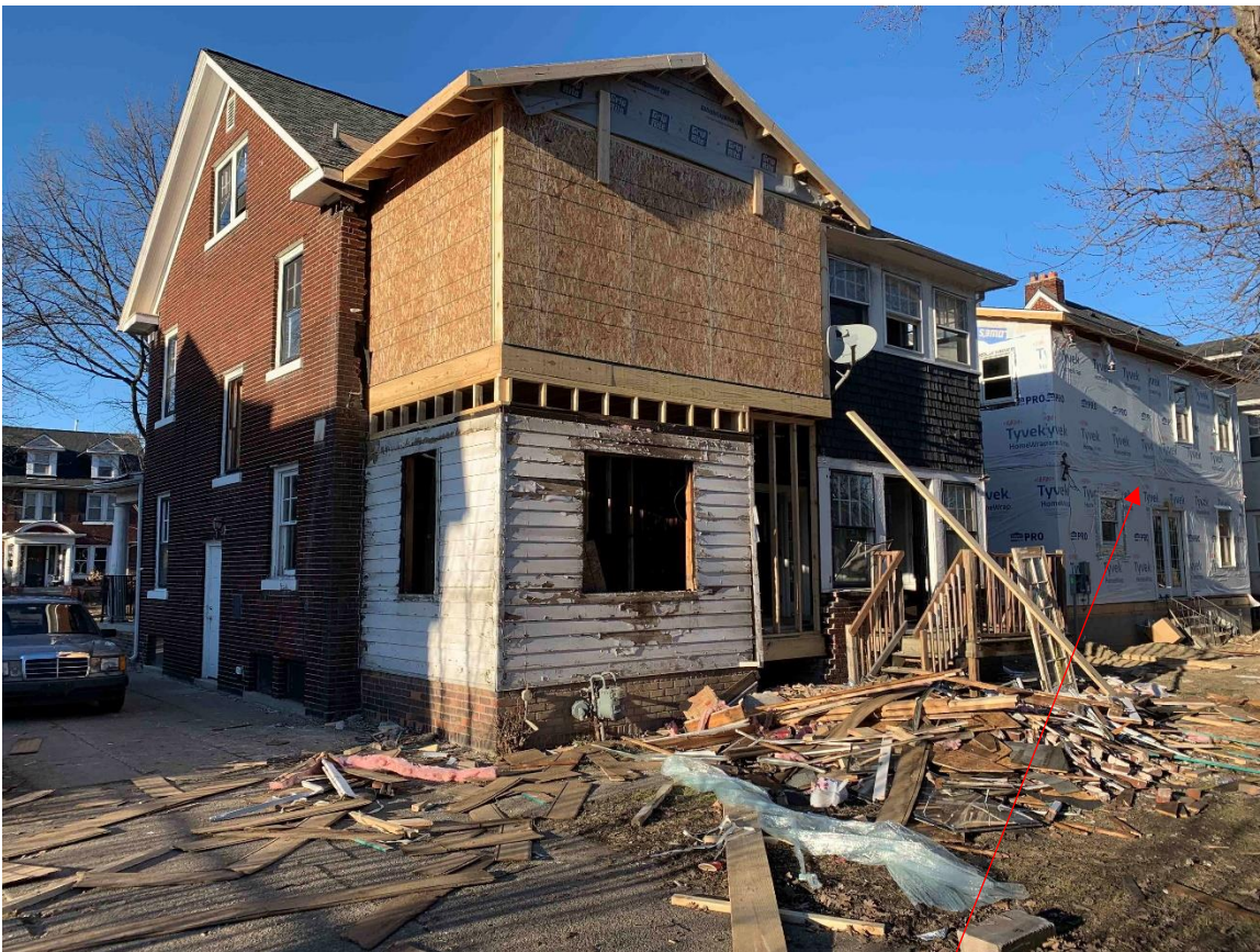
Photo showing home on 2/14/2024. Submitted by resident. Facing northwest, showing unapproved work at rear (outlined in yellow). Also, note that a new addition had been added to the rear of the home next door/1475 Longfellow without HDC review/approval. 1475 Longfellow is also owned by owner of 1485 Longfellow
