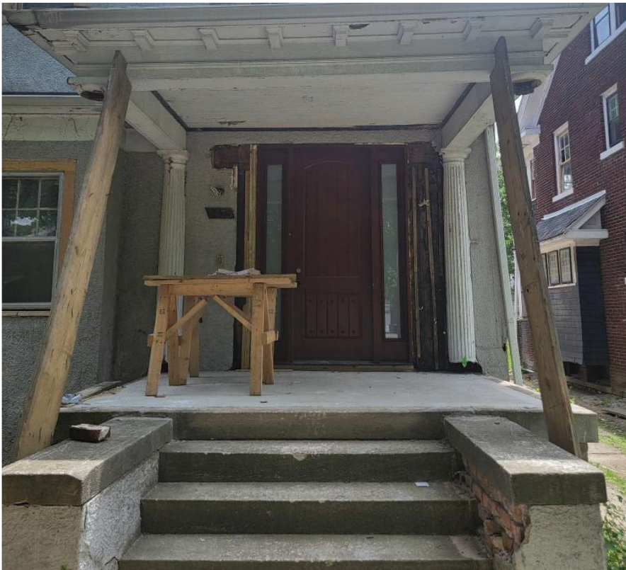
1475 Longfellow, current appearance of front elevation primary entrance. Photo provided by applicant. Detail of new front door and sidelites. Note that the historic fluted pilasters which flank the front door still remain.
