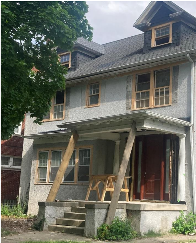
1475 Longfellow, current appearance of front elevation. Staff photo taken on 5/29/2024. Note that shutters, porch columns, and front door have been removed without HDC approval sometime between December 2023 and May 2024., after the property owner had received an approval from HDC staff for the replacement of the roof and repair of original windows.
