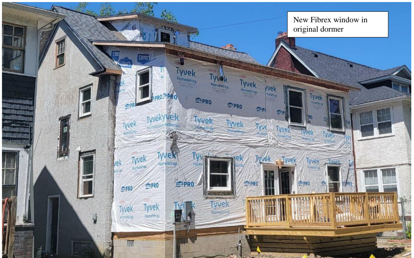
Rear elevation, showing unapproved addition, deck, and new window in original dormer. Facing northeast. Photo taken by the applicant.
