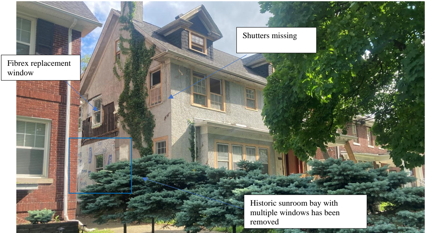
East elevation, staff photo taken on 5/29/2024. Note replacement window at second story. Also, the second story shutters and first story sunroom bay are no longer extant (see area outlined in blue). This work was completed without HDC approval
