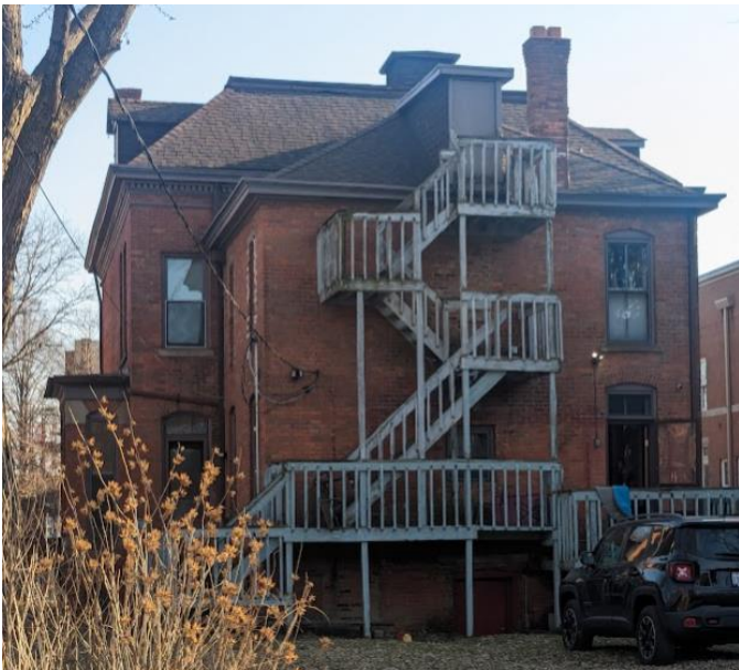
February 2024 photo by staff. Reduced window openings with non-historic windows are visible at the east (left of photo) elevation, second floor.
