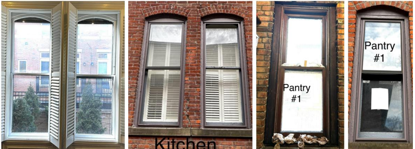
Three examples (interior and exterior views of each) of windows proposed for replacement; images from application, cropped by staff. Please see application for additional, higher-resolution photos.
