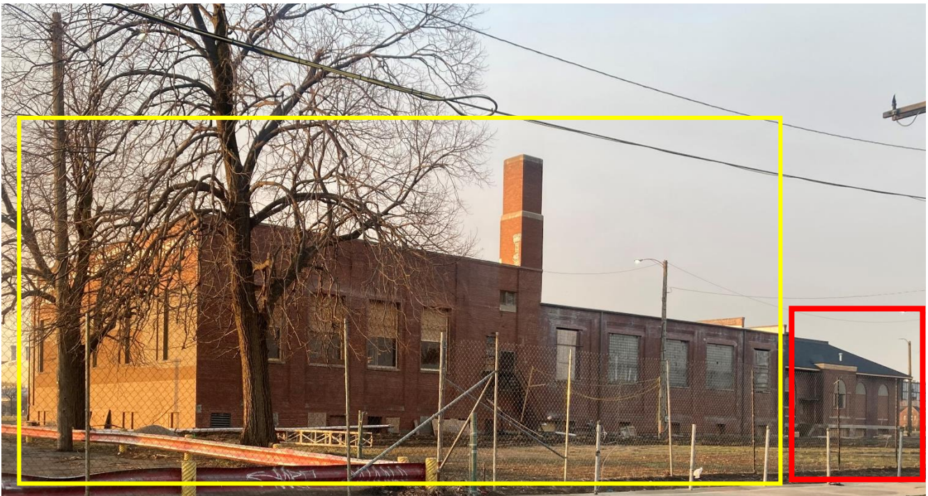
2900 St. Antoine current condition, facing southwest. 1917 original library wing, outlined in red and 1929 community/recreation center addition outlined in yellow. Staff photo taken 2/27/2024
