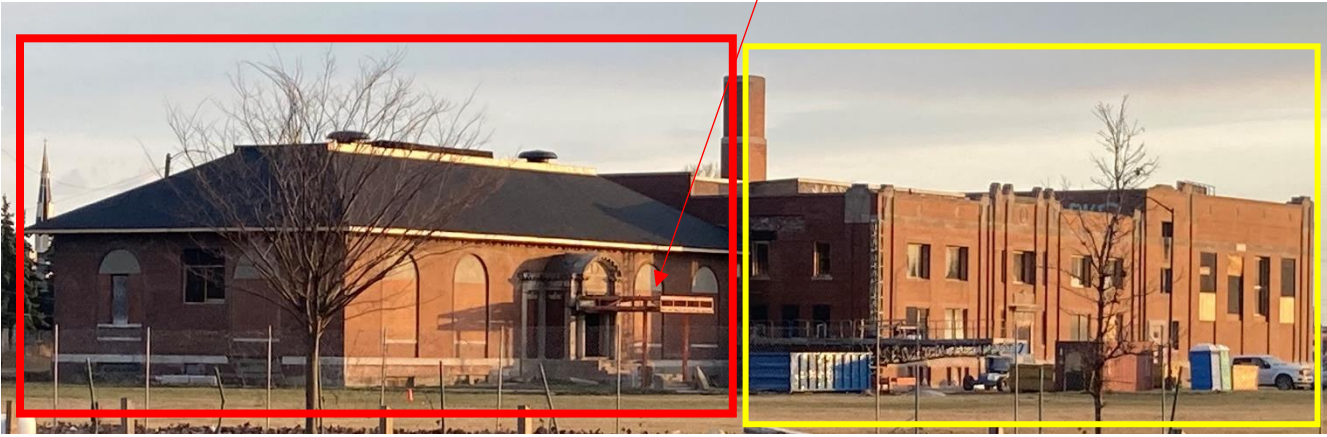
2900 St. Antoine, current condition, facing northeast. 1917 original library wing, outlined in red and 1929 community/recreation center addition outlined in yellow. Note the remaining steel framing at the 1917 wing's entry door. Staff photo taken 2/27/2024.
