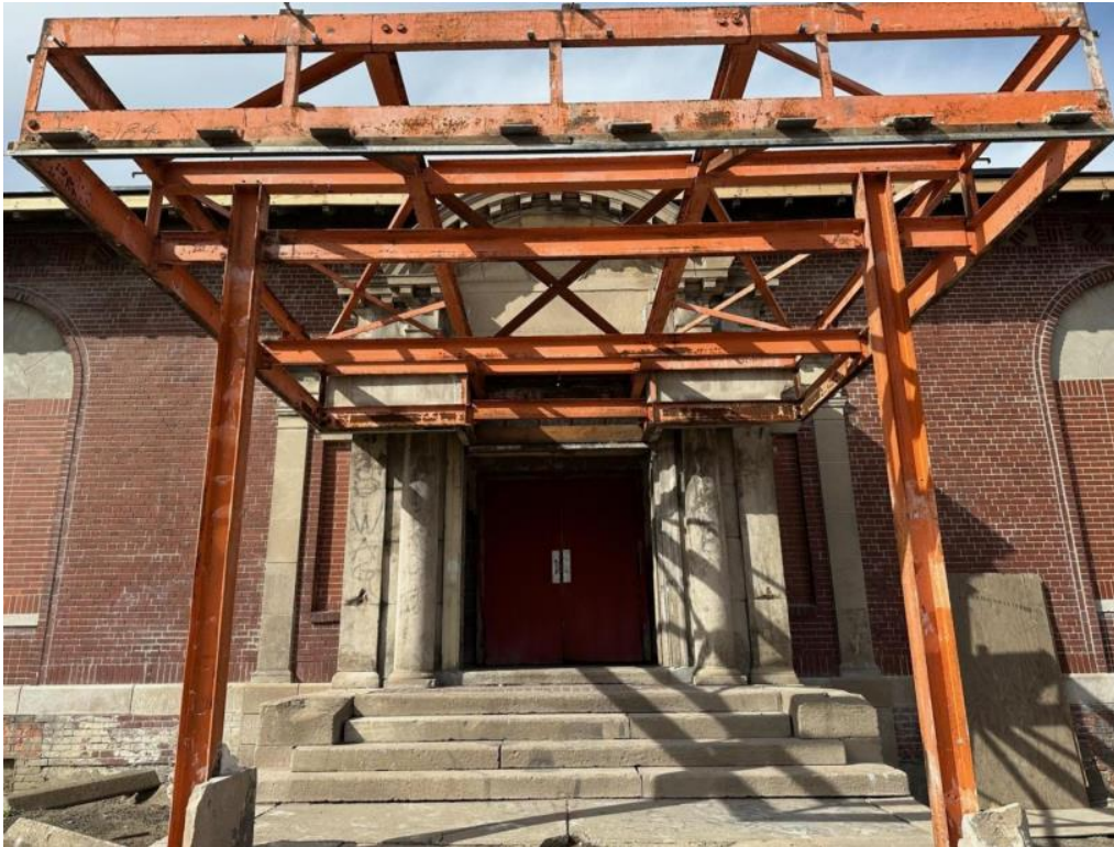
2900 St. Antoine, flat roof canopy after to the unapproved limestone cladding removal/current condition. Photo provided by applicant
