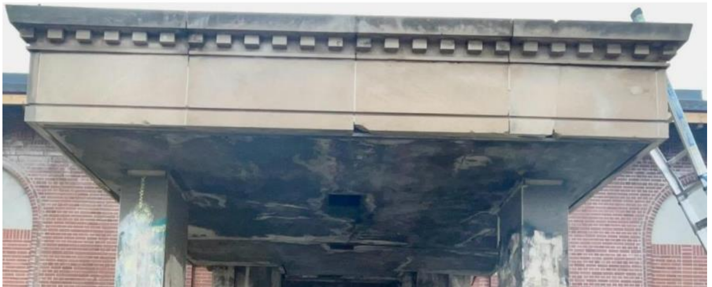
2900 St. Antoine, flat roof canopy prior to the unapproved limestone cladding removal. Photos provided by applicants
