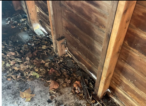
Interior baseboard damage of the garage.
