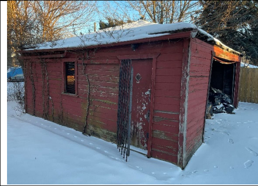
North elevation of garage showing wood damage along the foundation and roofline.
