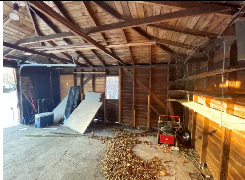
Interior roof and siding of the garage condition of the north, east and west sides.
