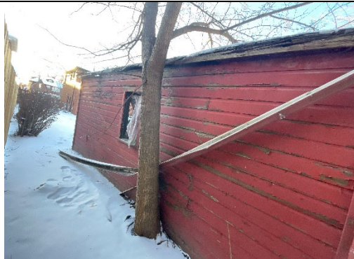
South side of garage, showing roof damage and non-historic mulberry tree, which is likely one of the sources of roof damage.
