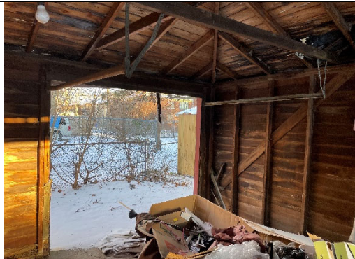
Rear door facing the alley, showing some roof damage.
