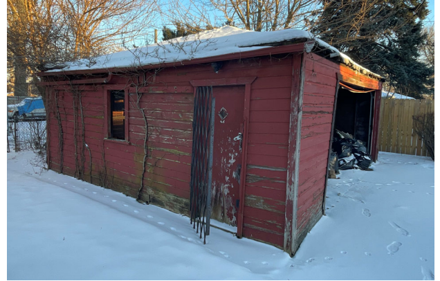
Site Photo 2, by Staff January 17, 2024: (West) front and side elevation of the garage.
