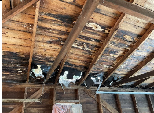
Garage roof and beam damage along south face area of the roof.
