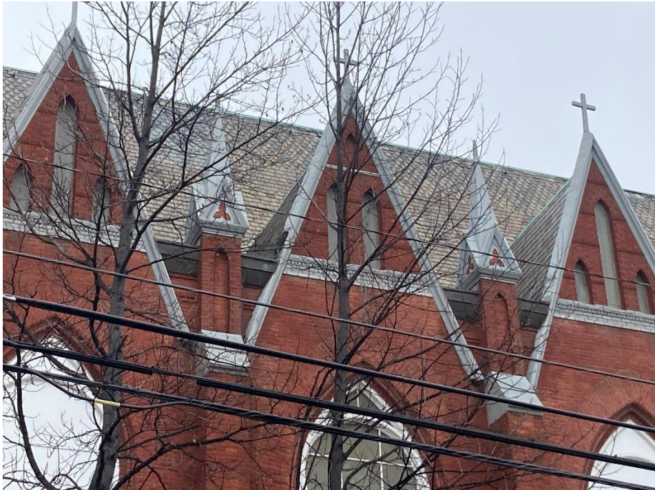
Current conditions, facing northeast, detail showing metal fascia with cross-shaped finials, metal spires with trefoil detailing, and copper gutters typical at roof. These elements will be removed in whole/throughout and will be replaced with new copper elements to match the existing. The slate near the ridgeline (i.e. the area of the decorative diamond pattern) is of a scalloped type/shape, while the remainder is a more typical square edged slate Staff photo taken 1/25/2024
