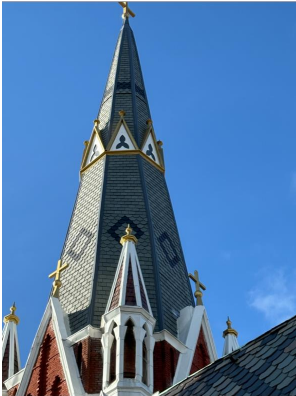
Spires showing recently installed Davinci synthetic slate roofing, photo provided by applicant
