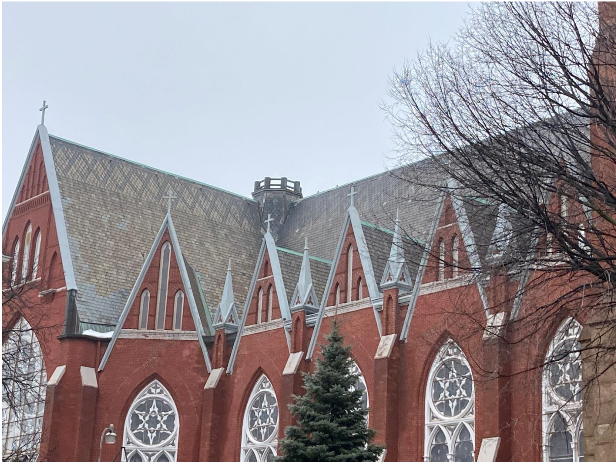
Current conditions, facing northwest, detail showing metal fascia with cross-shaped finials, metal spires with trefoil detailing, copper gutters, copper ridge caps typical at roof. These elements will be removed in whole/throughout and will be replaced with new copper elements to match the existing. Staff photo taken 1/25/2024
