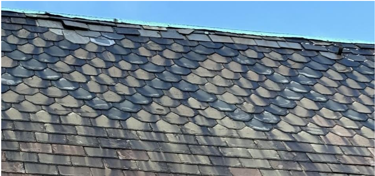
Scalloped shingles and diamond pattern at roof's ridgeline. Photo provided by applicant.
