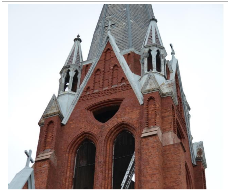
Photos provided by applicant, 2017, prior to steeple repair
