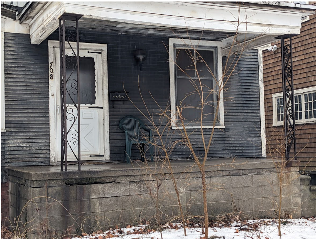
View of existing non-historic concrete block porch at front entrance. Staff has confirmed that the porch, including the incompatible 1970s-style support columns, was extant at the time of district designation in 1982 (not a violation). Staff photo, January 24, 2024.
