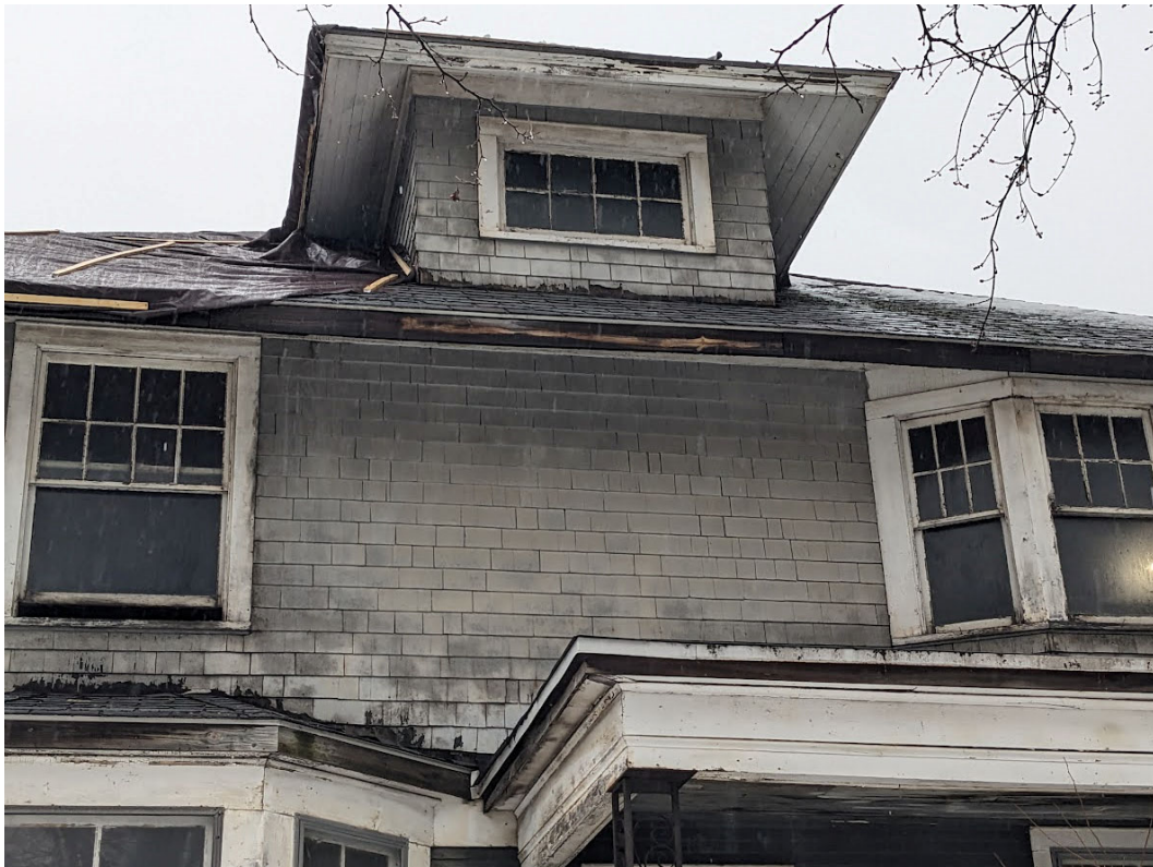
Detail view of second floor and dormer at front, showing historic materials and conditions. Staff photo, January 24, 2024.
