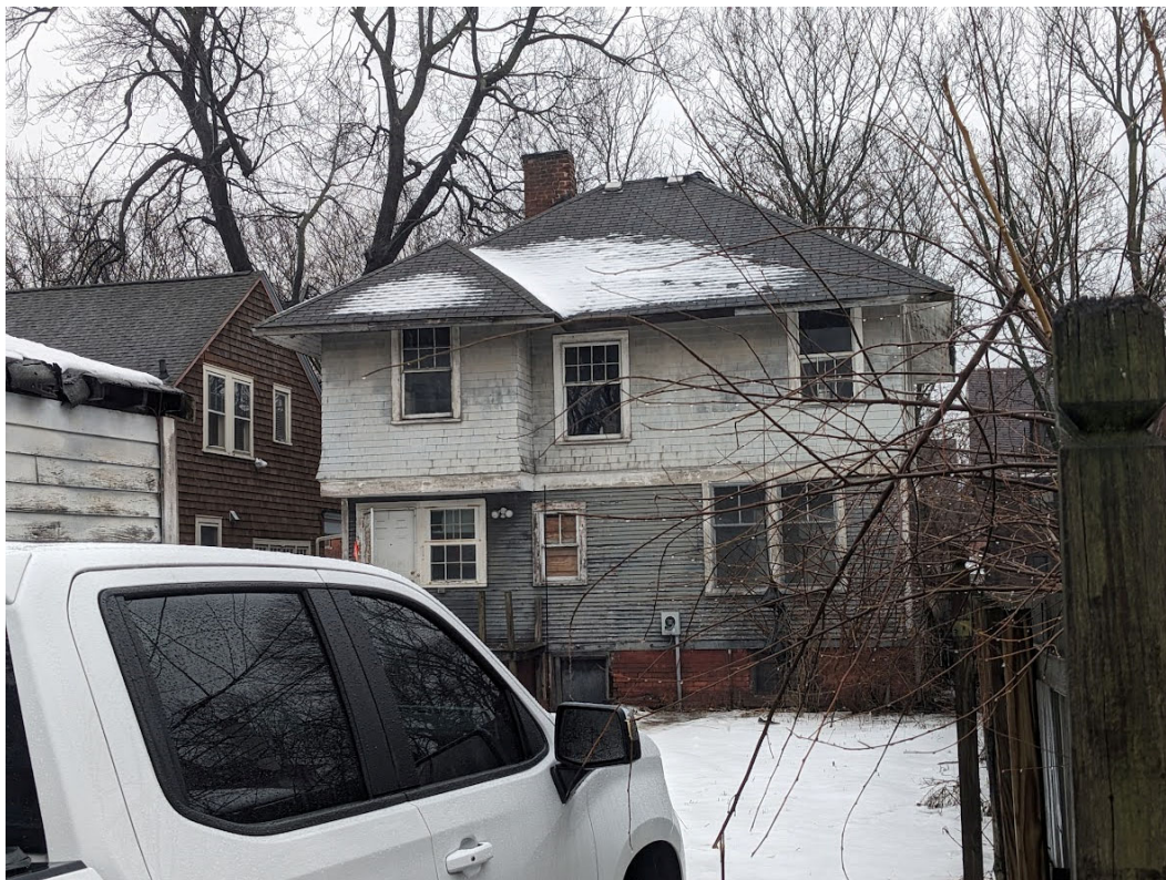
View of the rear elevation, from alley. Note the high level of historic integrity here, with original windows and historic siding fully wrapping the house. The pair of 2/1 windows at lower right are proposed for replacement with a sliding glass door. Staff photo, January 24, 2024.
