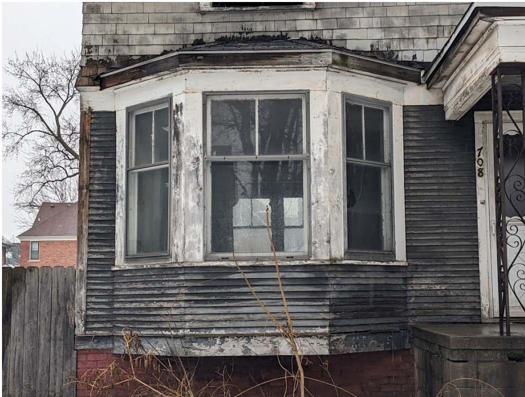
Detail view of 1 st floor bay window at front, showing narrow-exposure clapboard siding, original 2/1 windows, cedar shake at the second floor, and deterioration due to deferred maintenance. The 2/1 windows at the rear, proposed for removal, are partially visible in this view through the house. The incompatible porch is also partially visible at far right. Staff photo, January 24, 2024.
