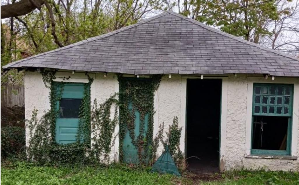
“Before” photo of garage, from April 22, 2022, garage repair application by previous owner.
