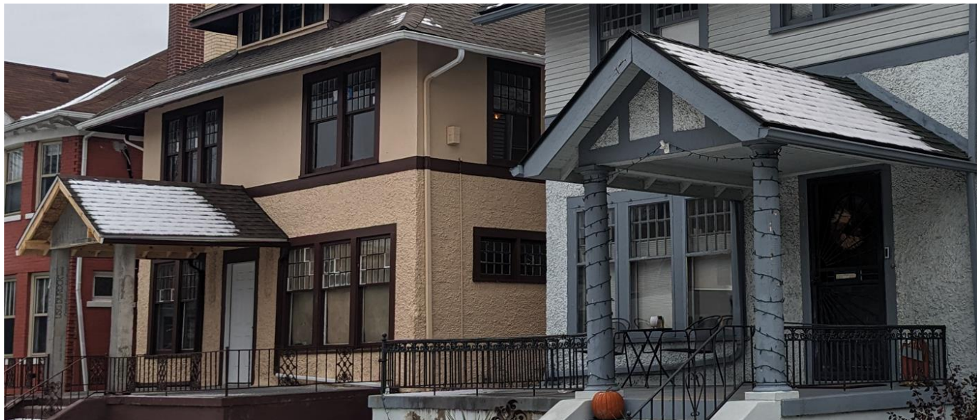
A side-by-side comparison of 859 Edison (left) and 867 Edison (right) highlights the architectural compatibility of the new porch. The work is nonetheless inappropriate (see “Issues,” below). November 2023 photo by staff.
