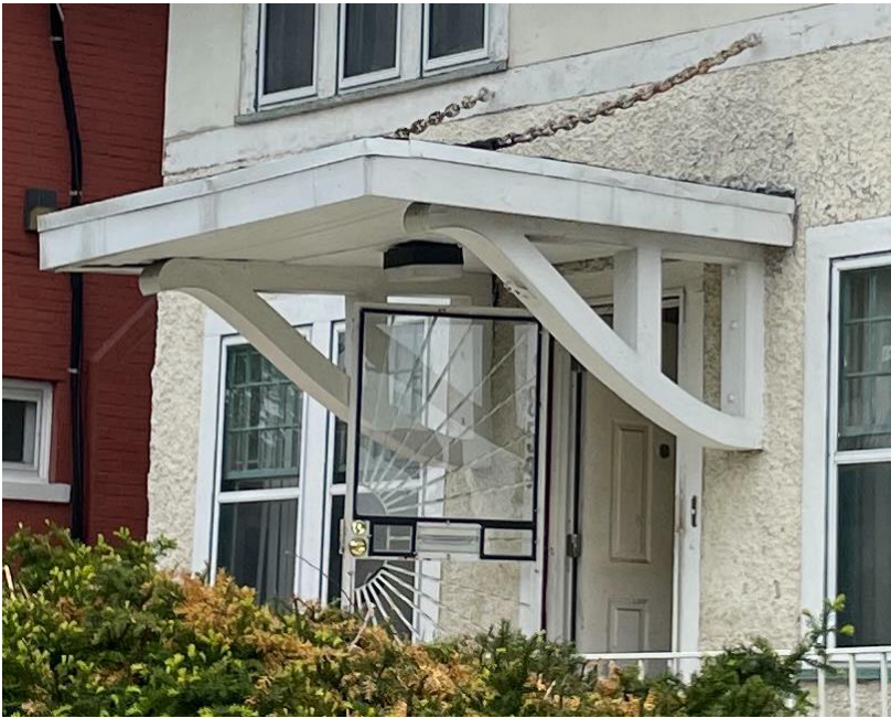
“Before” photo of porch roof. May 2022 photo by staff. (Photo was taken during a site visit pertaining to the security light, a separate scope item described below.)
