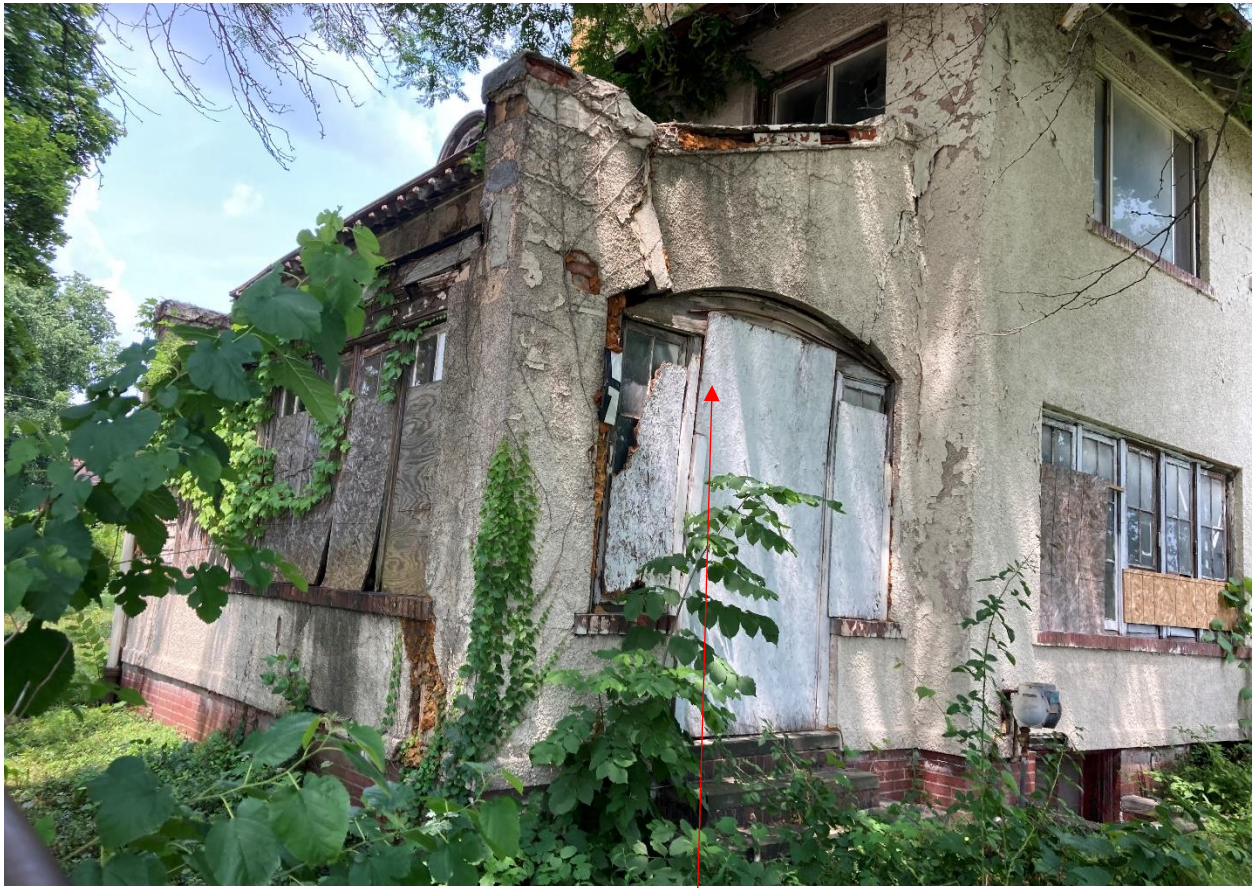
Facing northeast. The south wall shown here will be rebuilt to match the existing in materials and design with the exception that it will only include window openings
